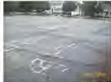
Basketball court and hopscotch play surface is in disrepair.
