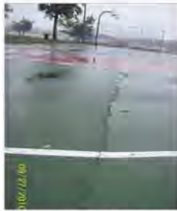
Cashman basketball court is cracked.
