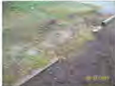
Approximately a dozen landscape ties need replacing.
