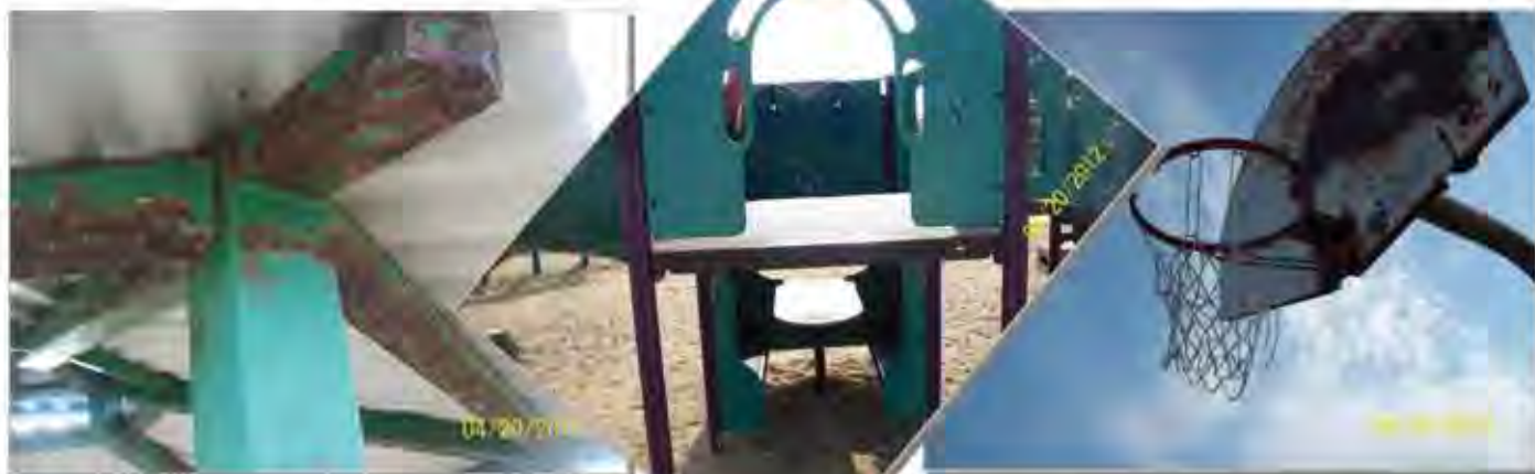
Top Left: Pavilion supports are badly rusted. Middle: Climbing ladder missing from central climbing structure Top Right: Basketball backboard needs replacement.
