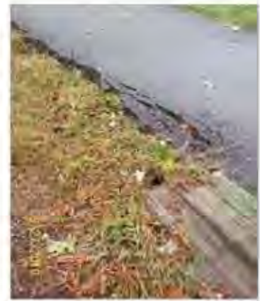
Missing landscape ties compromise the integrity of the asphalt walkway.
