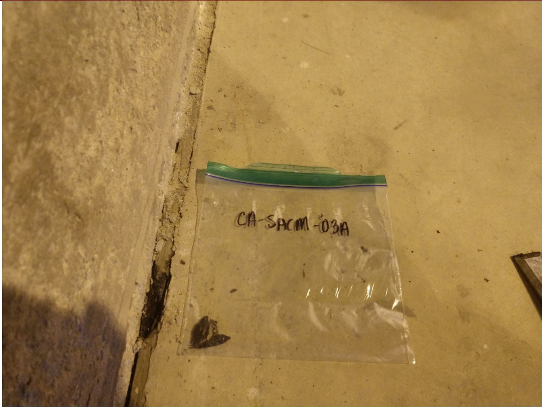
3. Material CA-SACM-03, expansion gasket found between the concrete floor and the concrete foundation wall
