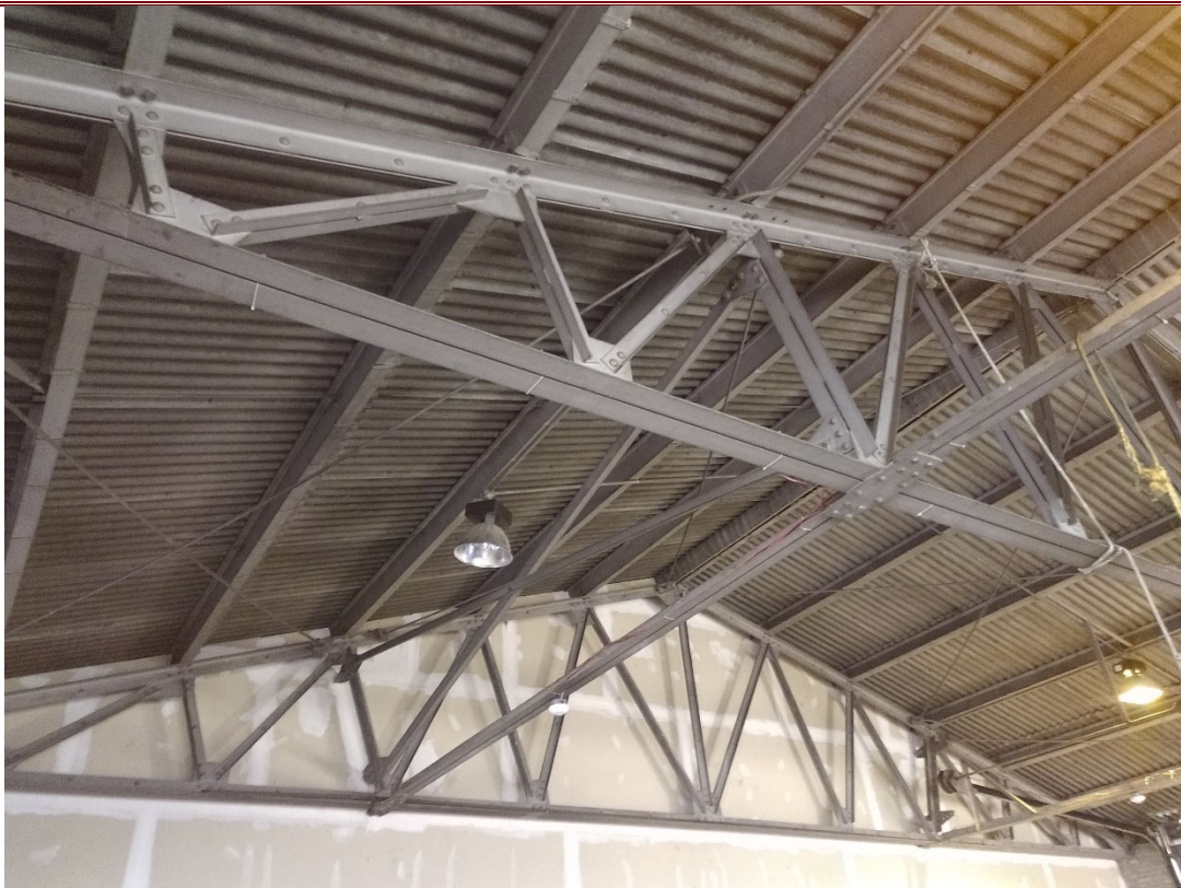
4. Material CA-SACM-04, corrugated transite panels in place on the building roof as viewed from below.
