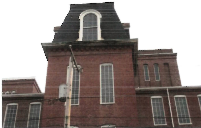
West elevation, detail of upper level of center stair tower, view east
