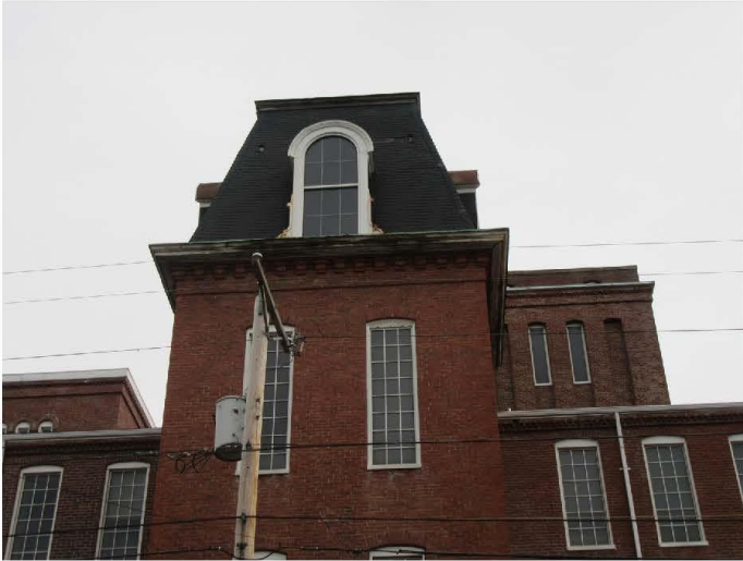
12. West elevation of 1866 building, detail of upper level of center stair tower, view east
