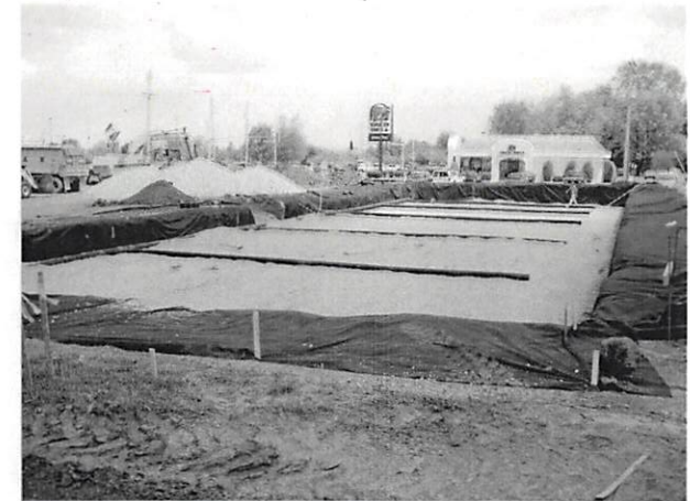
Place clean, crushed, angular stone foundation 6" (150 mm) min. Install underdrains if required. Compact to achieve a flat surface.
