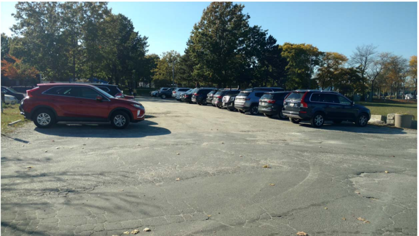
View of transition between paved and unpaved parking (East Lot looking West)
