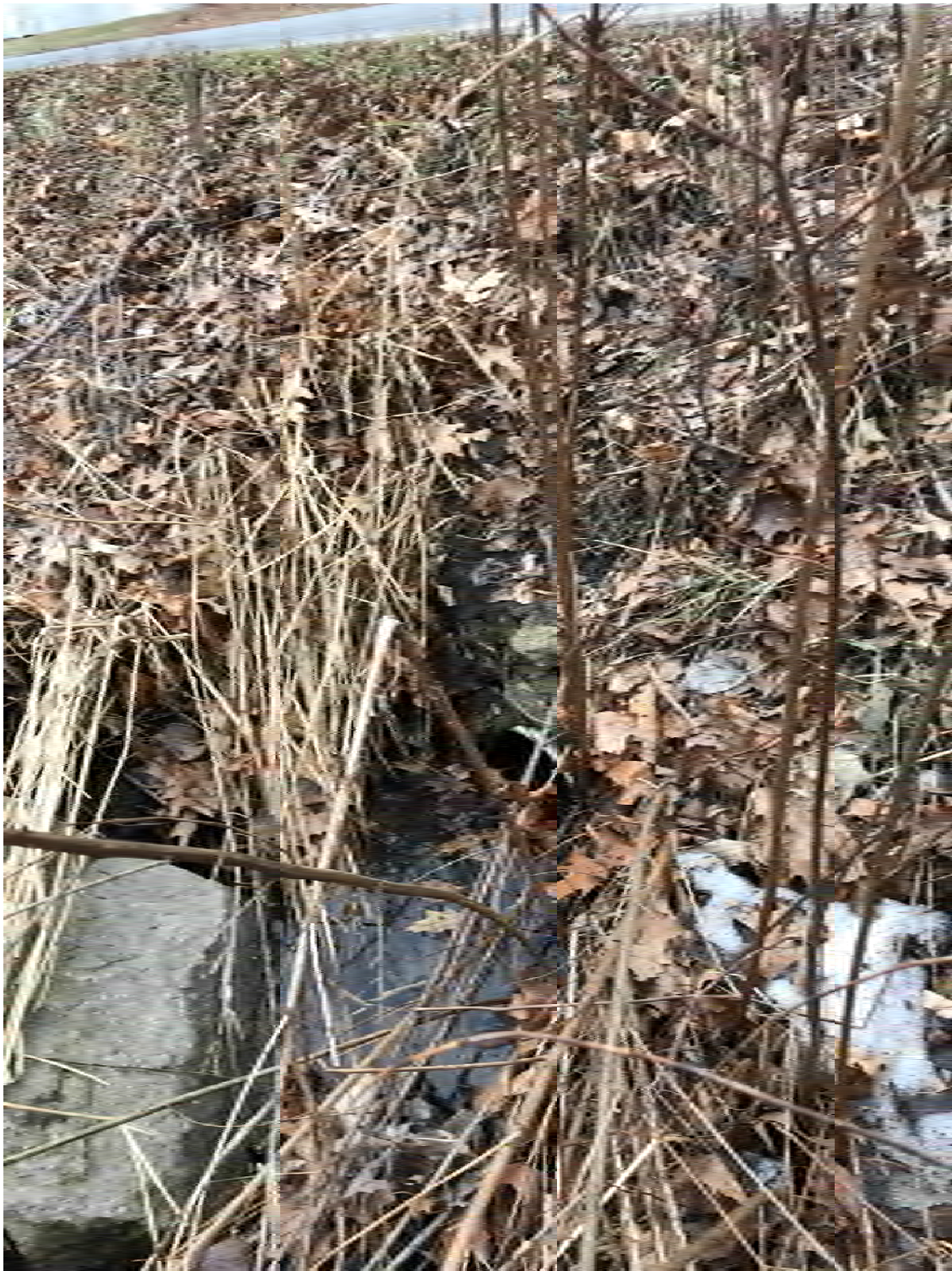
Figure 3: Drainage outlet into the bordering wetland
