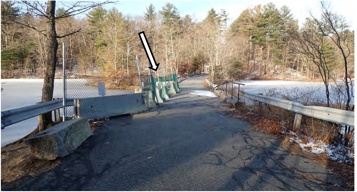
Photo #1: View northwest of Plummer Spring Rd, Newburyport facing Middle St, West Newbury over the Upper Artichoke Reservoir. Arrow indicates the failed section at the southern end of the roadway, directly over the bridge which is closed for public safety.
