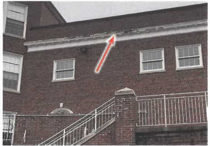
PHOTO 20: Paint deterioration throughout wood cornice at East and West wings of school.
