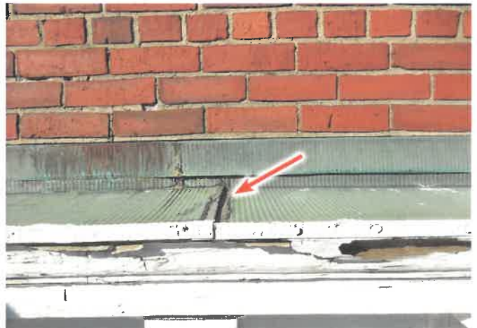
PHOTO 24: Opened solder joints due to rilled copper expansion, in absense of expansion joints.
