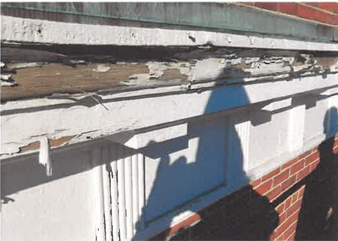
PHOTO 21: Peeled paint throughout East and West wing wood cornices.
