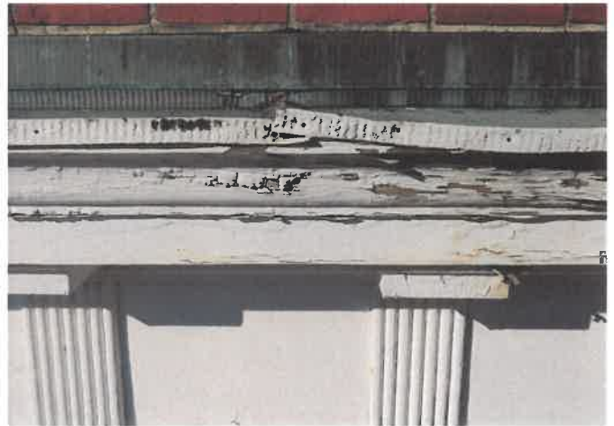
PHOTO 22: Failed solder joints and warped rilled copper at East and West wing wood cornices. Face-nailed hem is a poor detail.
