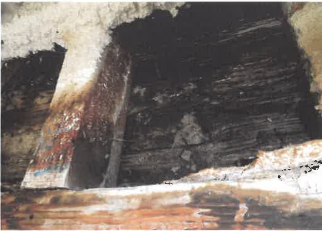
PHOTO 19: Water damage rot on cupola sheathing as seen from inside of cupola.
