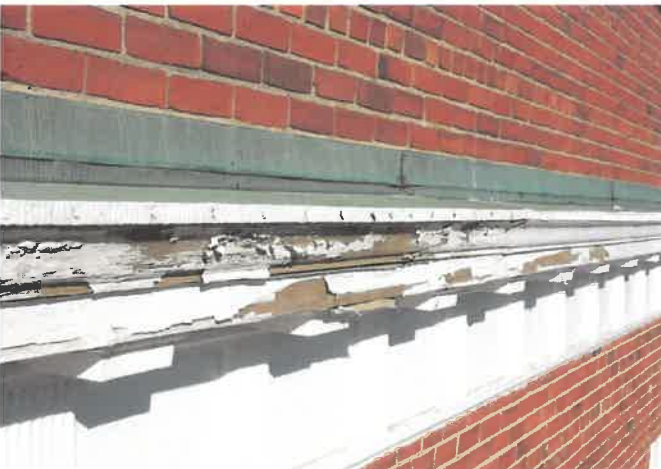
PHOTO 23: Face-nail rilled copper at East and Wing wood cornices has open joints due to temperature expansion.
