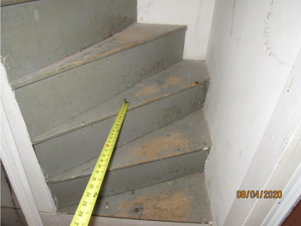
Photo 12 Stairs to attic are steep and difficult to climb
