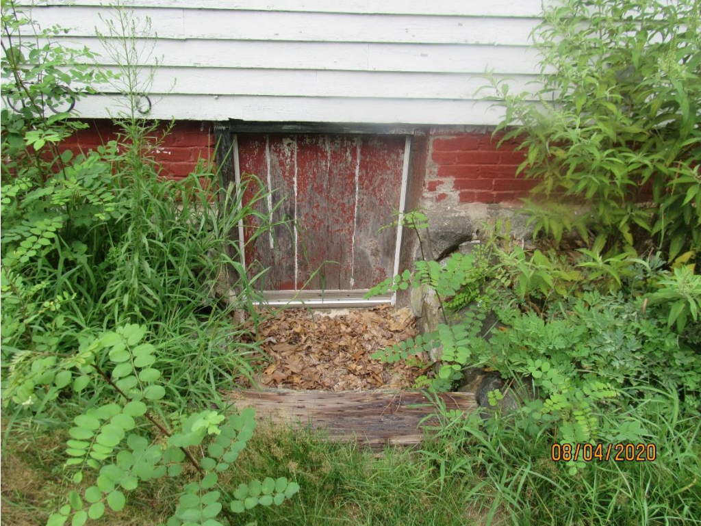
Photo 5 Exterior stairs uncovered and allow water intrusion into basement
