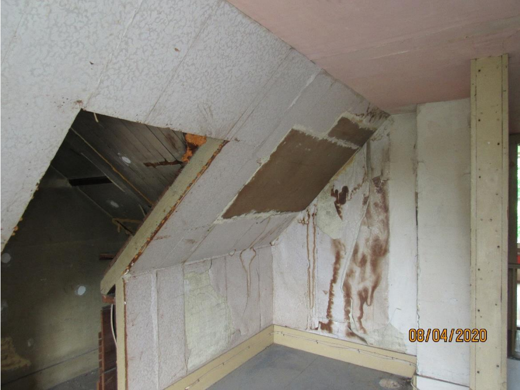
Photo 10 Lack of attic headroom
