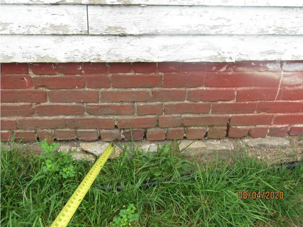
Photo 3 Brick and mortar deterioration on the West side foundation
