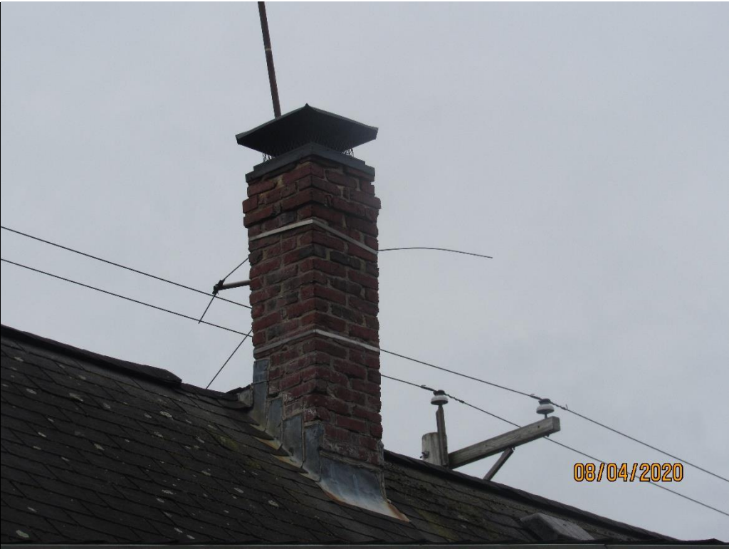
Photo 2 Deteriorated chimney bricks and aged roof shingles
