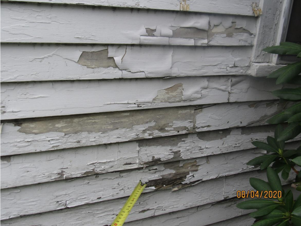
Photo 1 Deteriorated exterior clapboards
