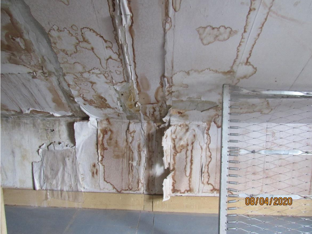
Photo 6 Moisture intrusion throughout the interior rooms
