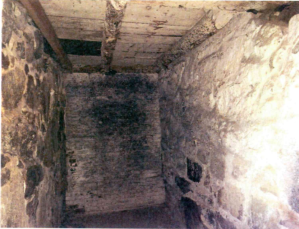
10. Basement condition – June 2015
