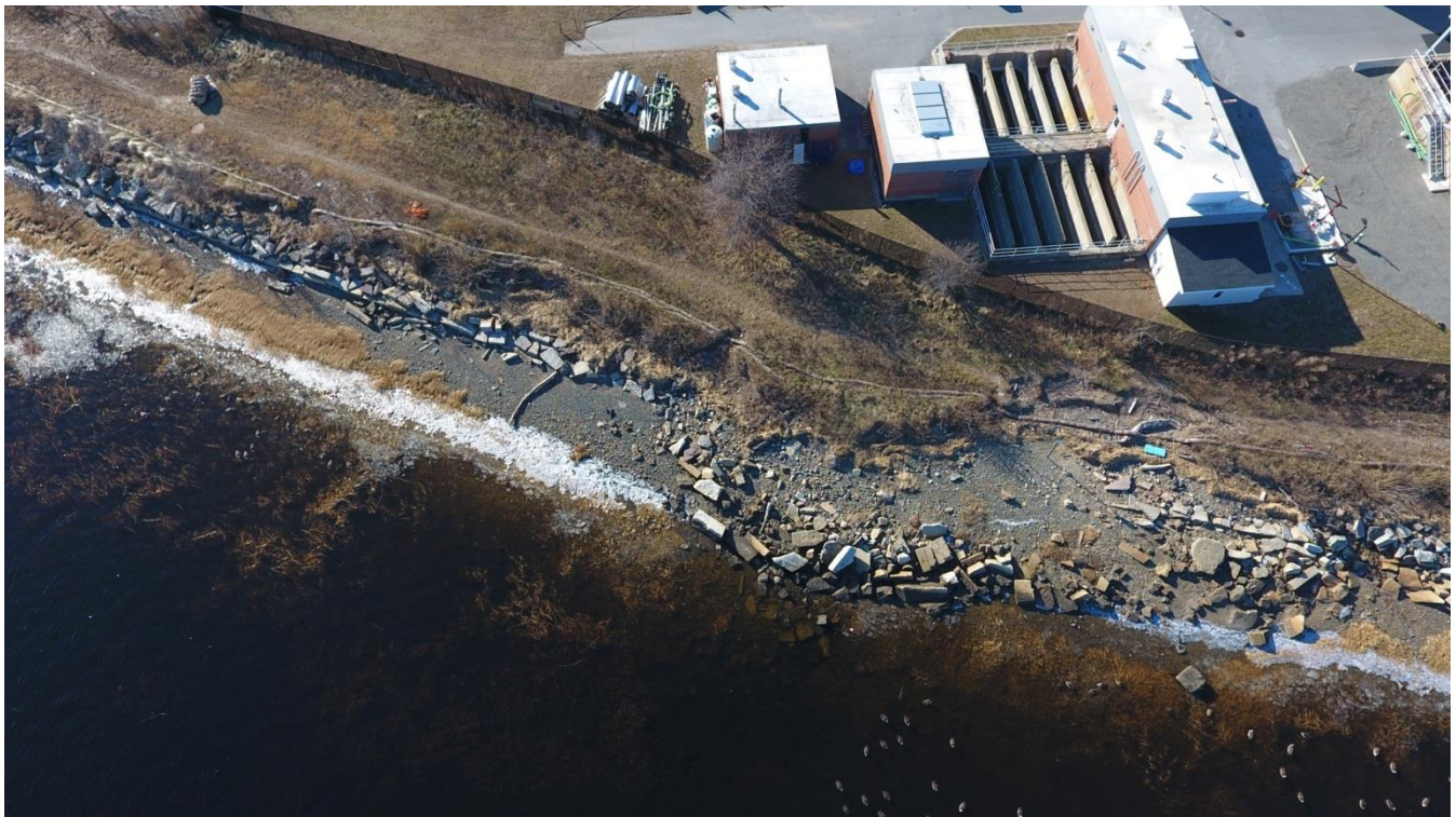
Aerial photo of eroded/scoured shoreline along riverfront trail corridor
