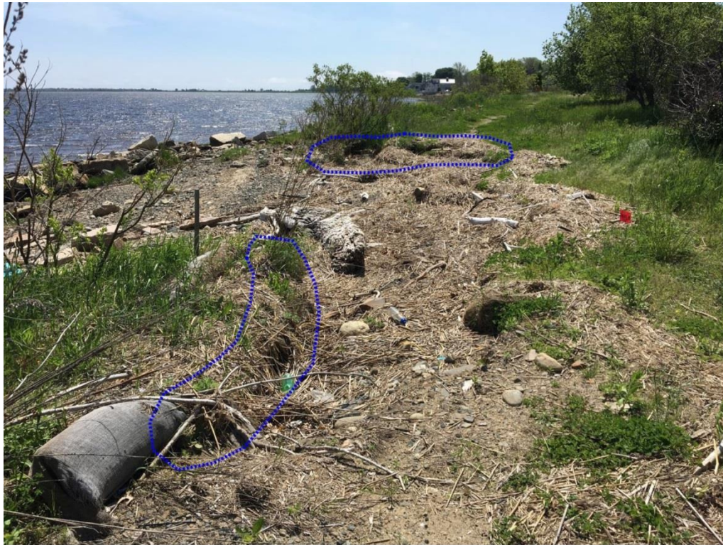
Debris from storm surge across riverfront trail corridor – eroded areas circled
