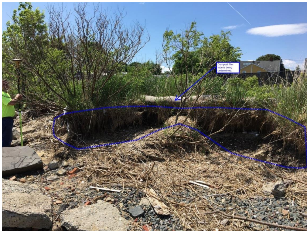
Scoured riverbank of trail corridor – eroded areas circled
