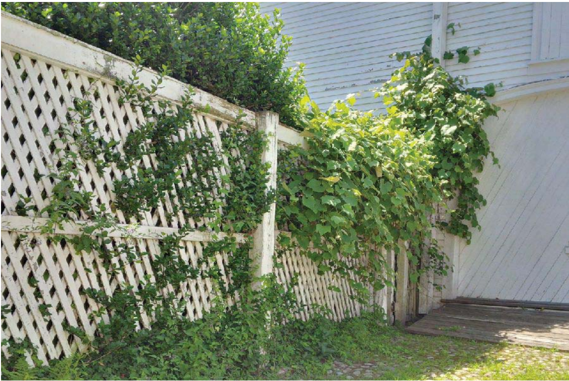
Alley looking towards Carriage Barn: Shows grapevine and holly shrub over lattice fence
