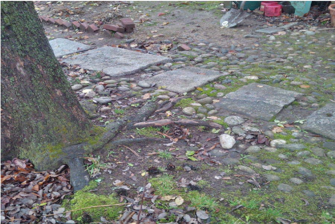
ON6: Detail photo of Orchard and Nursery path showing encroaching tree roots
