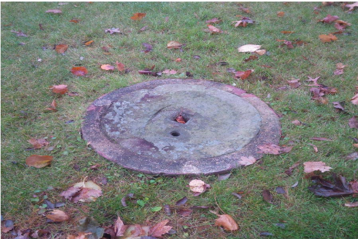
LY10: Detail view of manhole (well cover) at southeast side of Laundry Yard
