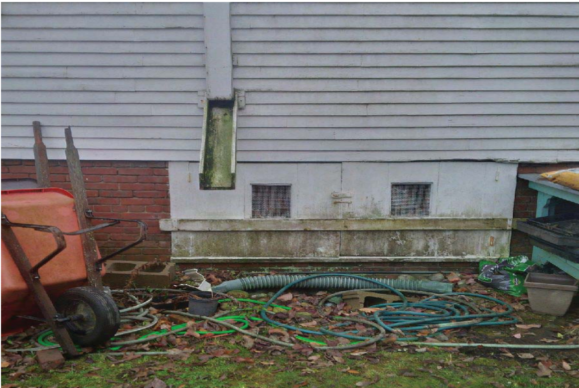
ON14: Northeastern side of Barn structure; view of gutter and hardware materials
