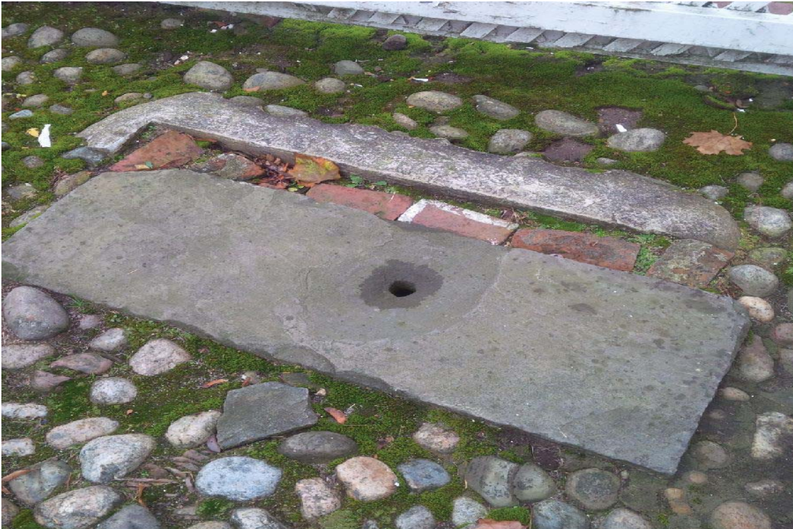
CY12: Close up of pump location in Courtyard
