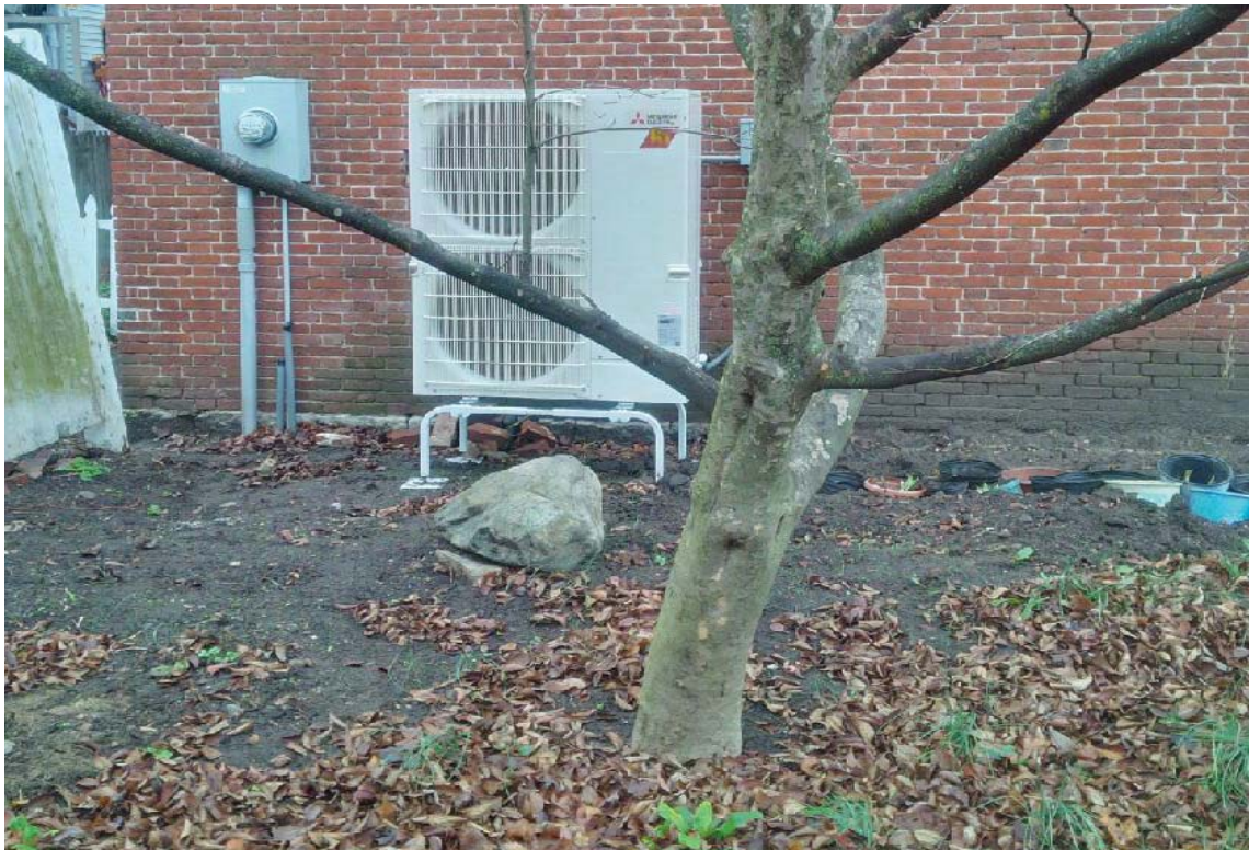
ON11: View of ventilation fan and utilities at western corner of Perkins Printing Building
