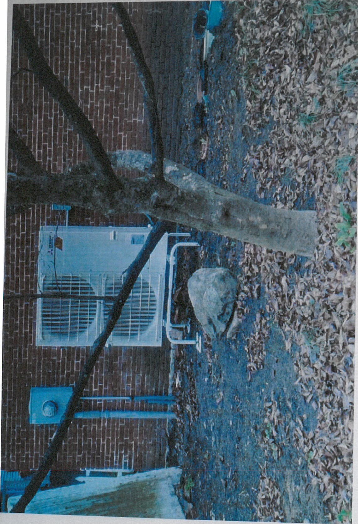
ON11: View of ventilation fan and utilities at western corner of Perkins Printing Building
