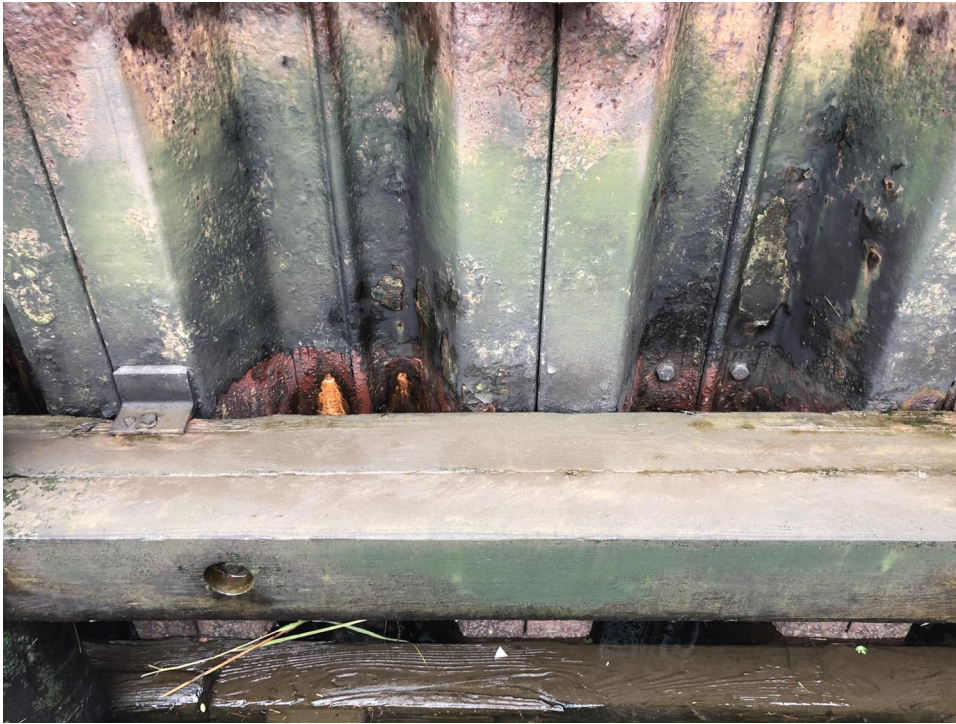
Existing Center Embayment – Missing bolts
