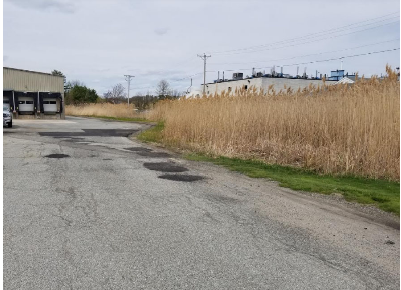
View of Phragmites invasion and damage to the adjacent driveway
