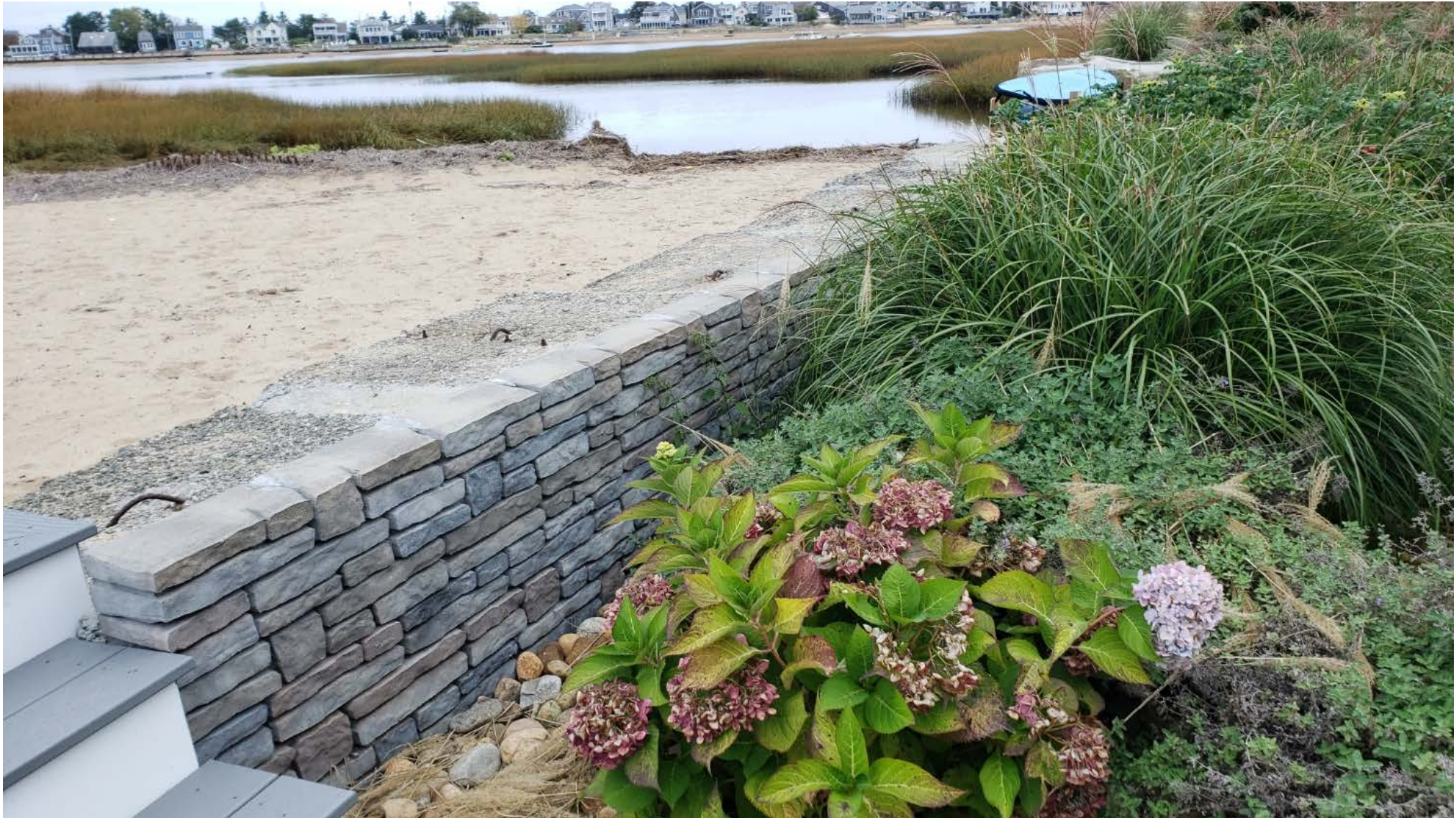
The above photo shows the imitation stone facing added to the existing concrete blocks.
