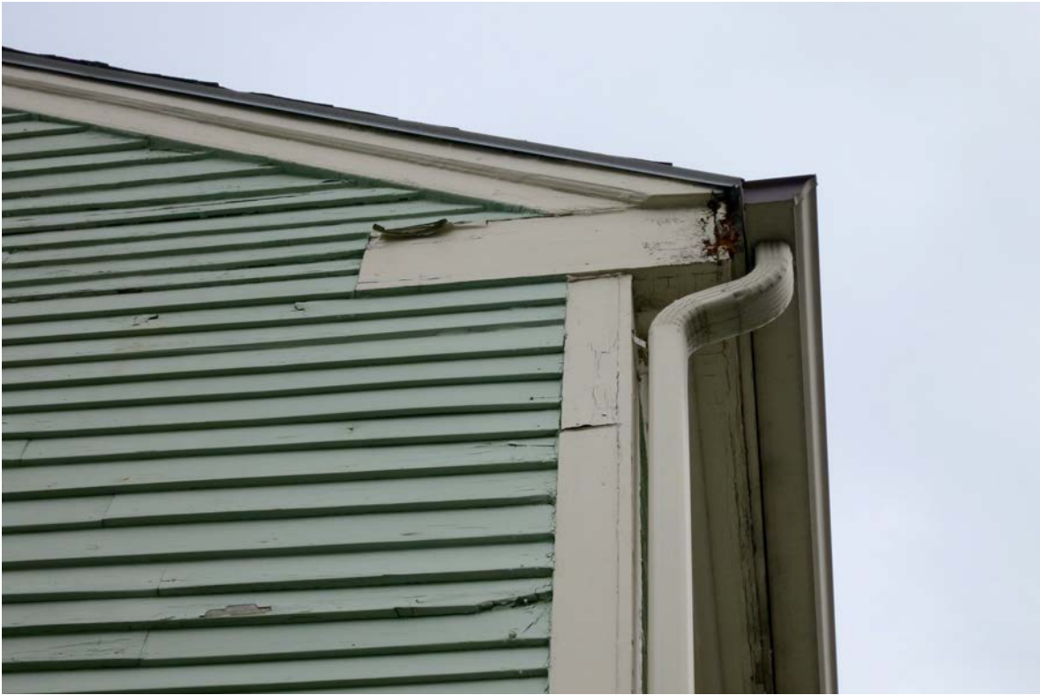
14_View southeast showing northwest elevation - detail of corner board, fascia, and return at gable
