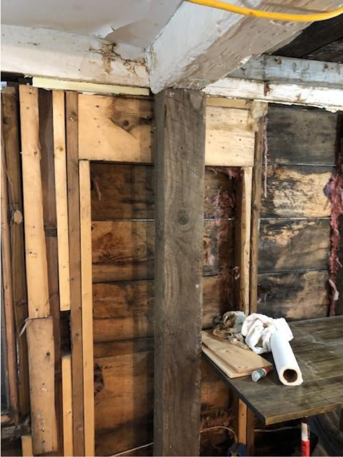
This is a center beam that was damaged by moisture penetrating through from the outside 25 years ago and had to have supports put in under the interior and exterior beams.
