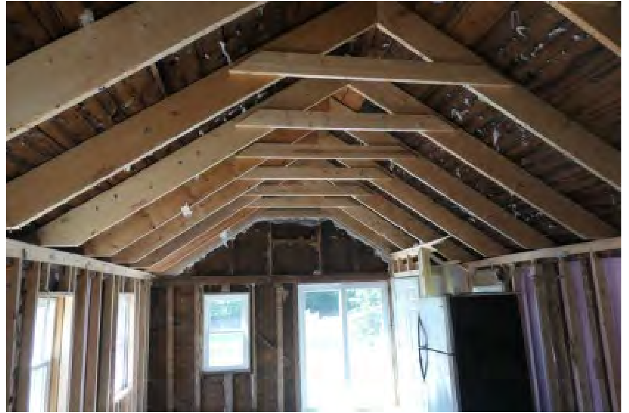
Second floor: Collar ties set too high, which induces too much stress in rafters. Also, the rafter seat cuts at the wall plate are too severe, resulting in overstress in shear.
