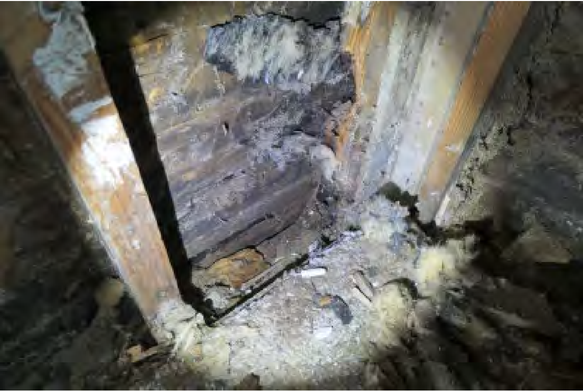
Interior view of rot and deterioration of rear wall of addition.
