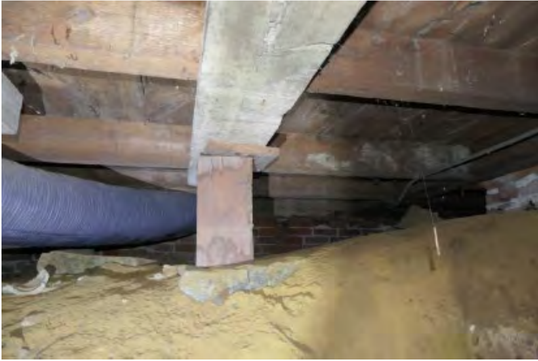
In crawl space under addition: wood column set on unstable stone.
