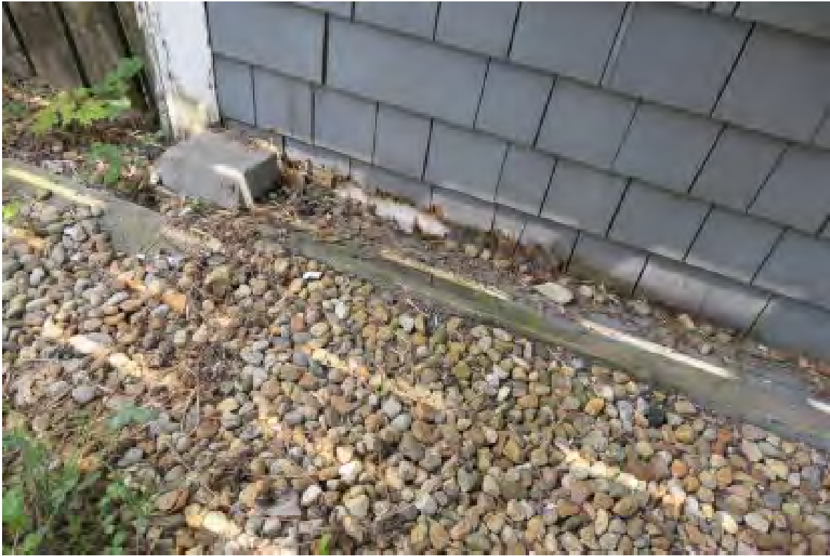
Rot of siding and sheathing at base of rear wall of addition due to grade too high.
