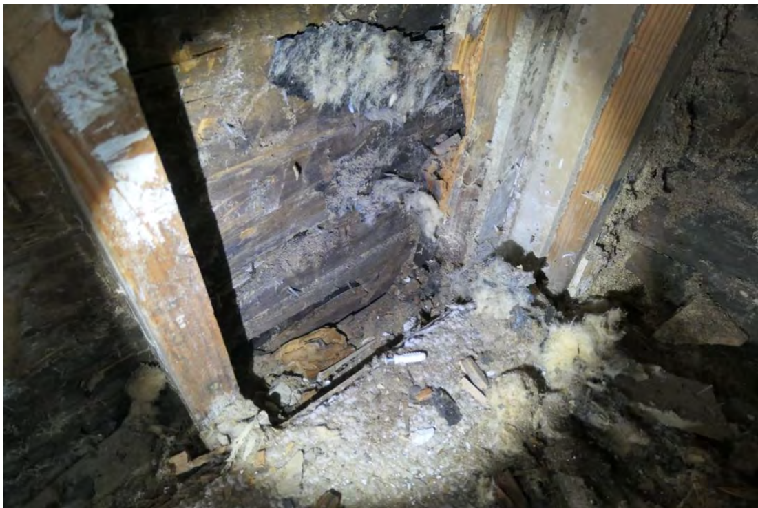
Interior view of rot and deterioration of rear wall.
