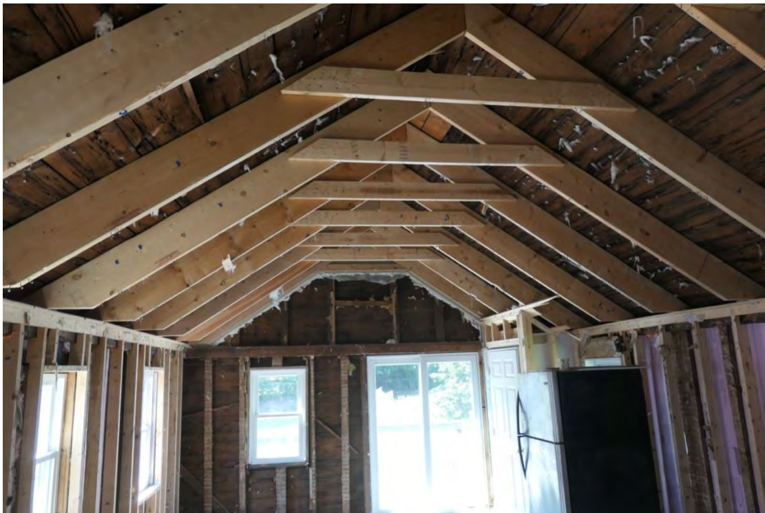
Collar ties set too high, which induces too much stress in rafters. Also, the rafter seat cuts at the wall plate are too severe, resulting in overstress in shear.
