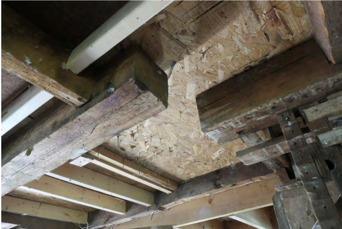
Second-floor framing: beams cut off, resulting in an unsafe condition.
