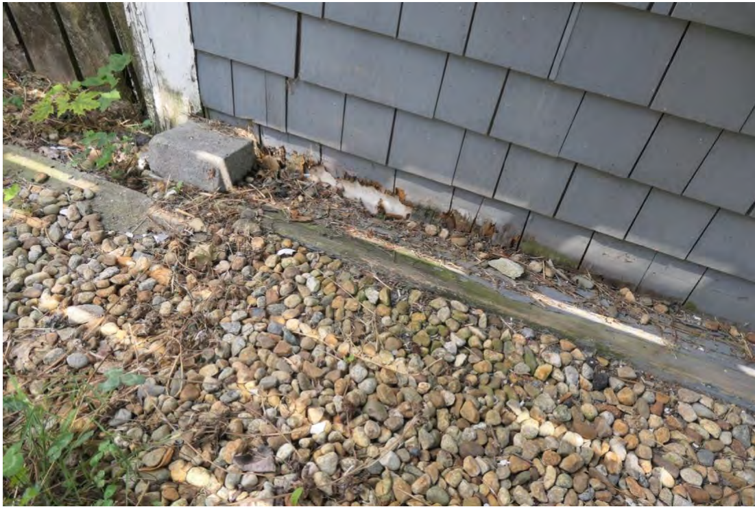
Rot of siding and sheathing at base of rear wall due to grade too high.
