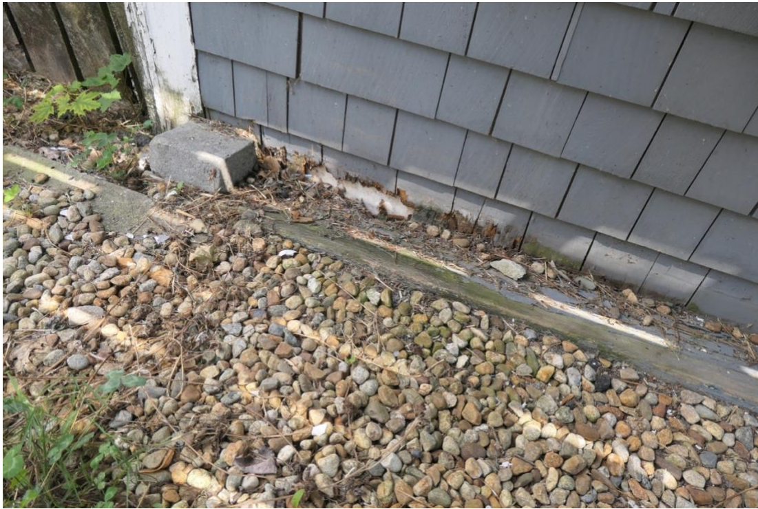
Rot of siding and sheathing at base of rear wall due to grade too high.
