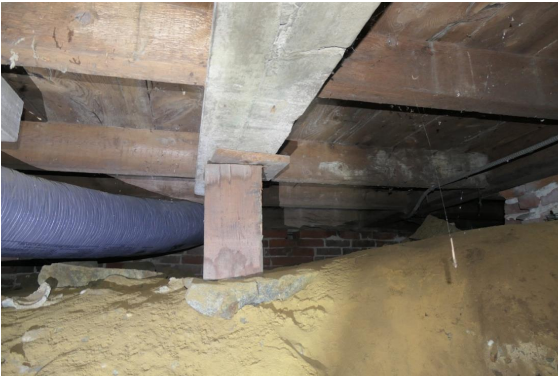
In crawl space: wood column set on unstable stone.
