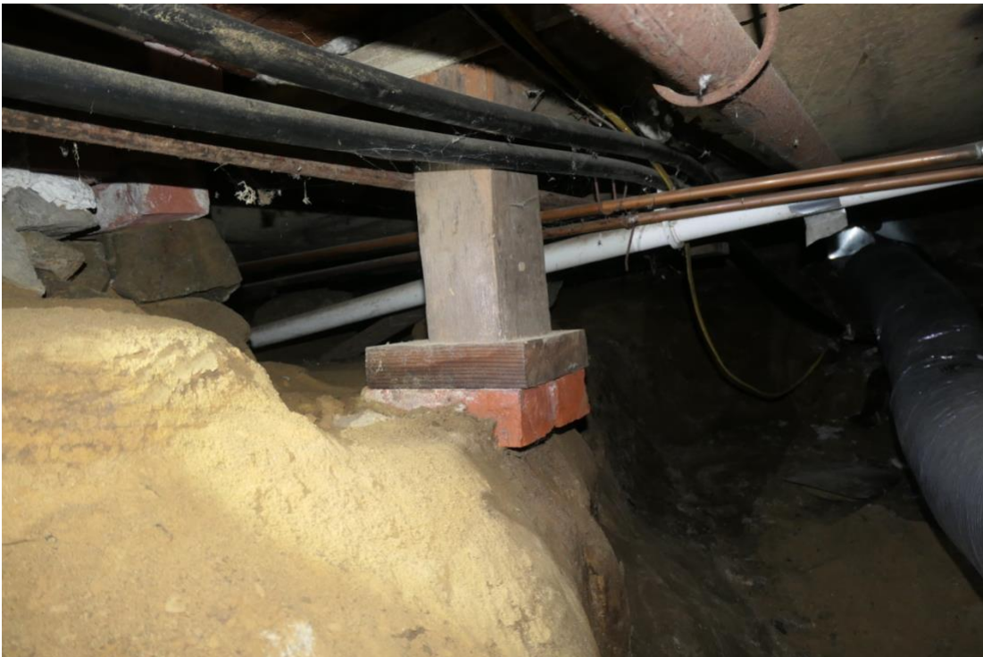
In crawl space: wood column set on unstable wood/ brick footing.
