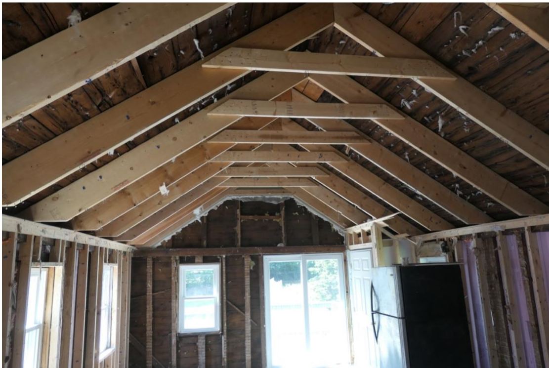
Collar ties set too high, which induces too much stress in rafters. Also, the rafter seat cuts at the wall plate are too severe, resulting in overstress in shear.
