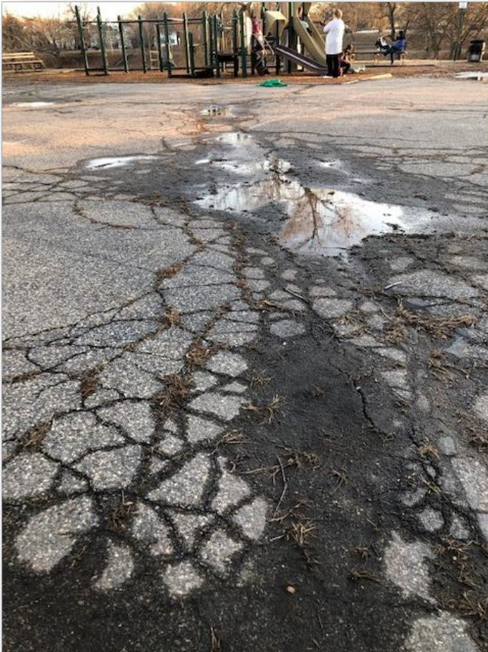
The asphalt basketball court at Bartlet Mall is badly cracked and uneven rendering it an eyesore, a hazard as a play surface, a barrier to accessing the park and nearly unusable for playing basketball.
