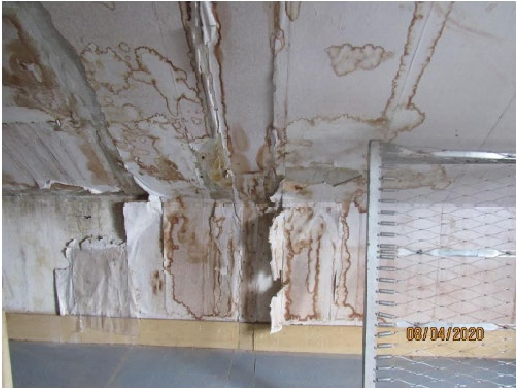
Photo 6 Moisture intrusion throughout the interior rooms
