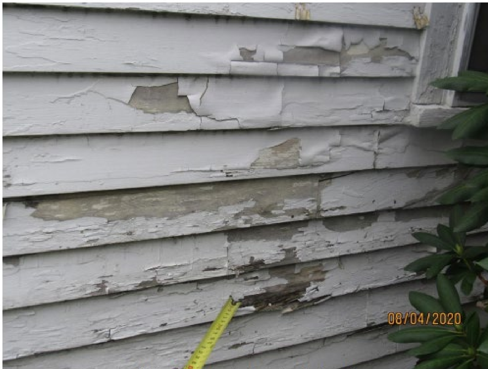
Photo 1 Deteriorated exterior clapboards
