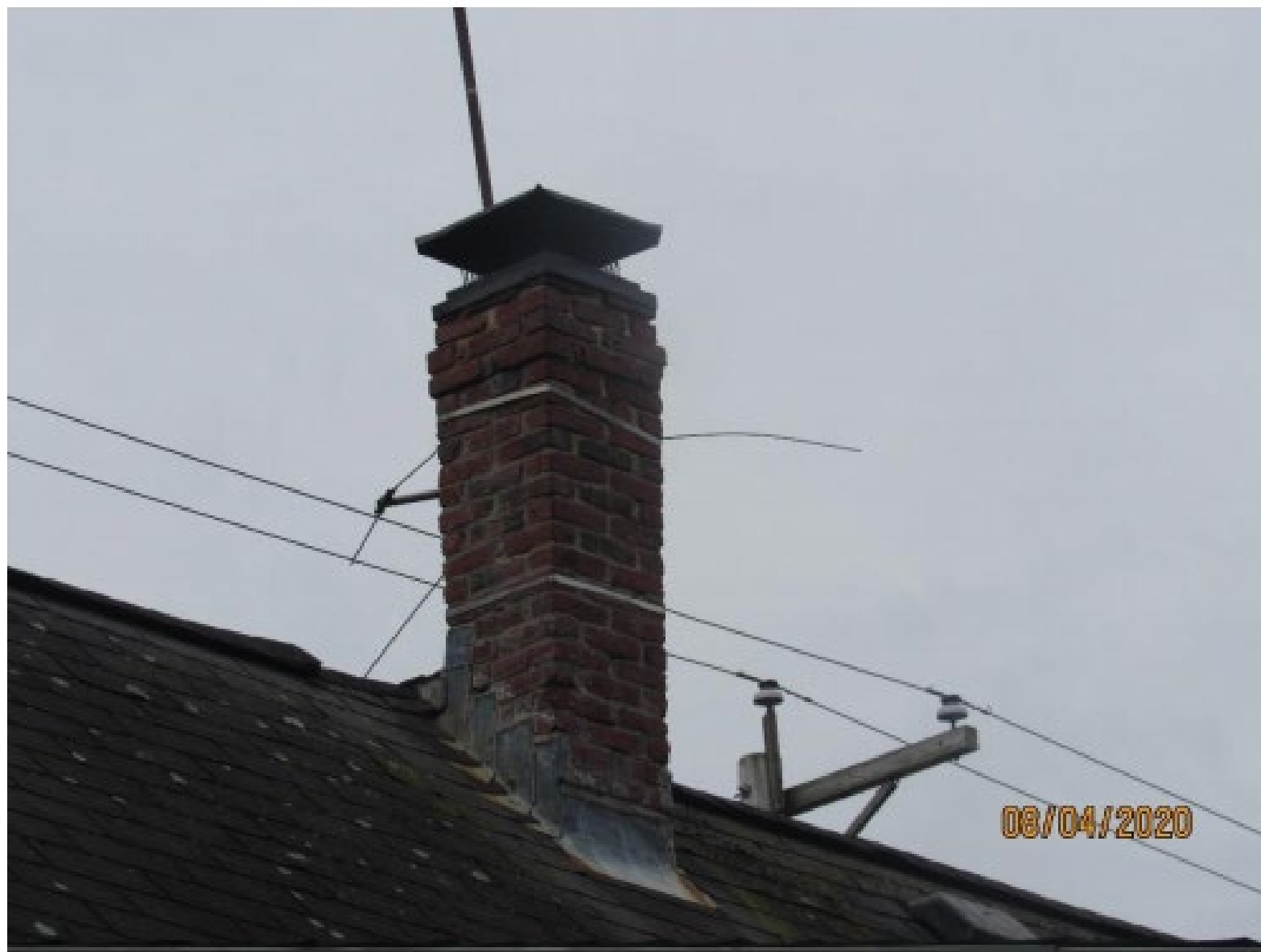
Photo 2 Deteriorated chimney bricks and aged roof shingles
