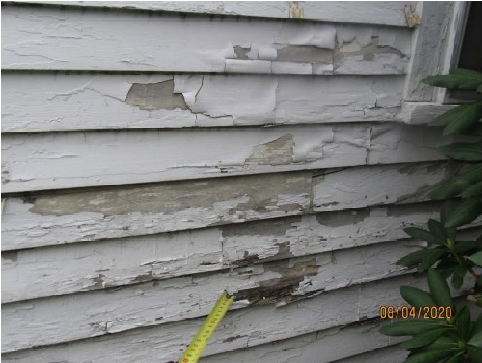
Photo 1 Deteriorated exterior clapboards
