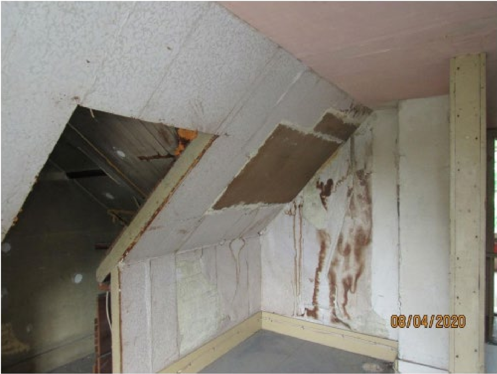
Photo 10 Lack of attic headroom
