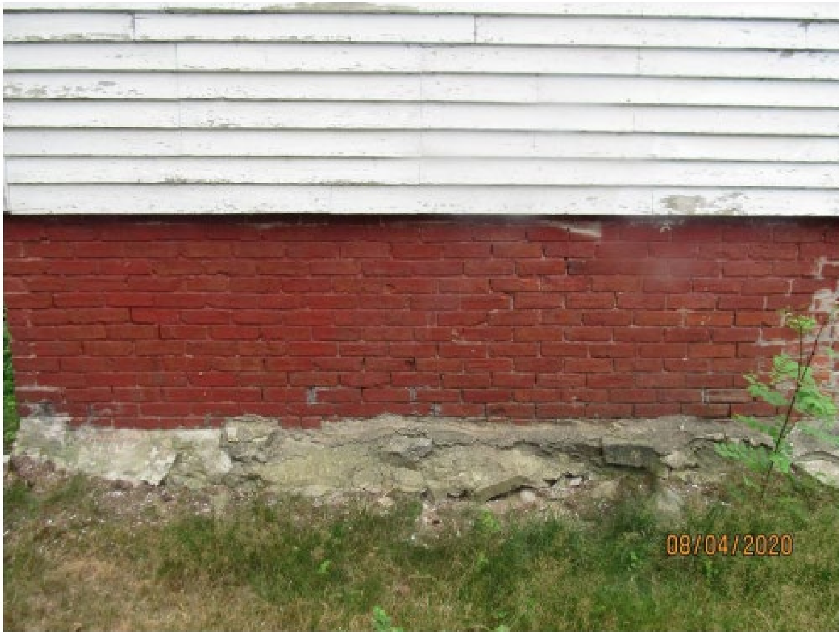
Photo 4 Fieldstone and brick wall deterioration on the North side foundation wall
