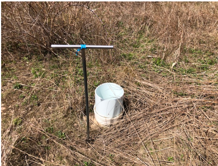
Riser Pipe in Stormwater Basin
