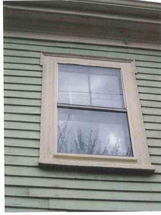
11_View northeast showing principal facade (northwest elevation) - detail of second floor window at south end
