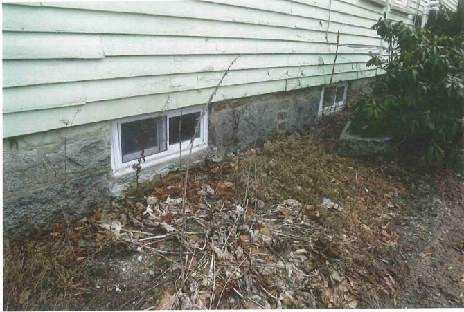
16_View southwest showing northeast elevation - detail of foundation to ell and basement windows
