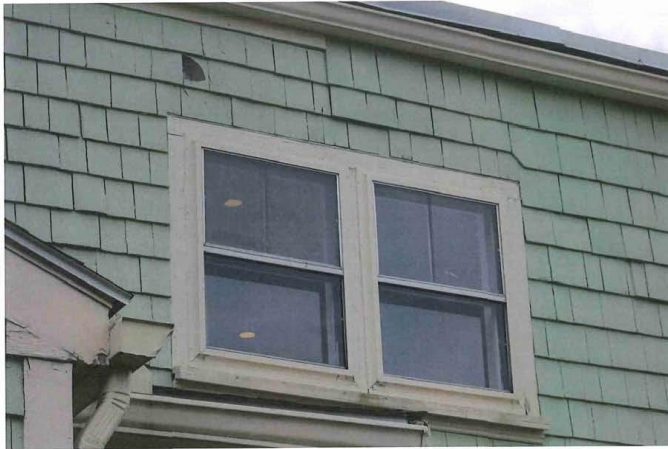
25_View southwest showing rear (southeast) elevation - detail of central bays at second floor
