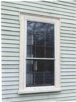
10_View northeast showing principal facade (northwest elevation) - detail of first floor window at south end
