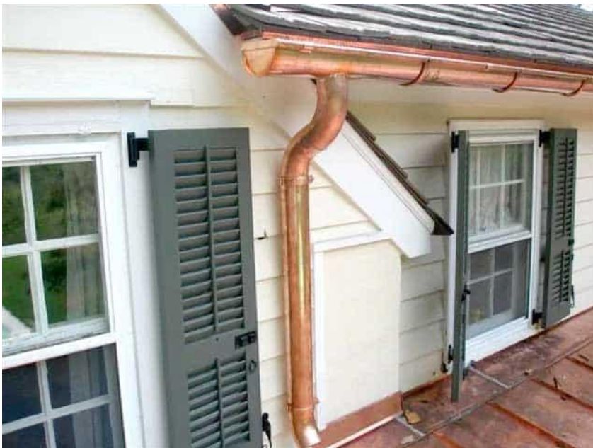
Figure 7 – Examples of Gutters and Downspouts
