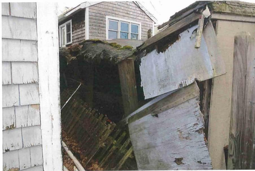
31_View northwest showing rear (southeast) elevation of deteriorated shed
