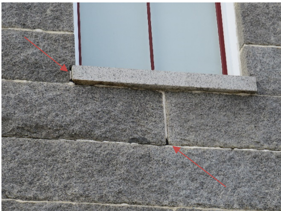
18. East façade window A3 – mortar loss at sill and vertical joint beneath
