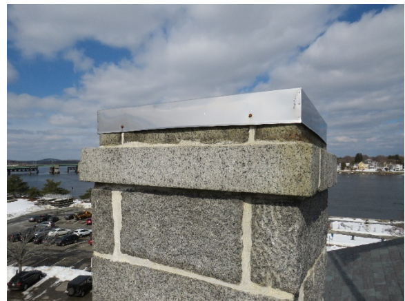
15. Northwest chimney cap – ferrous metal Tapcon screws
