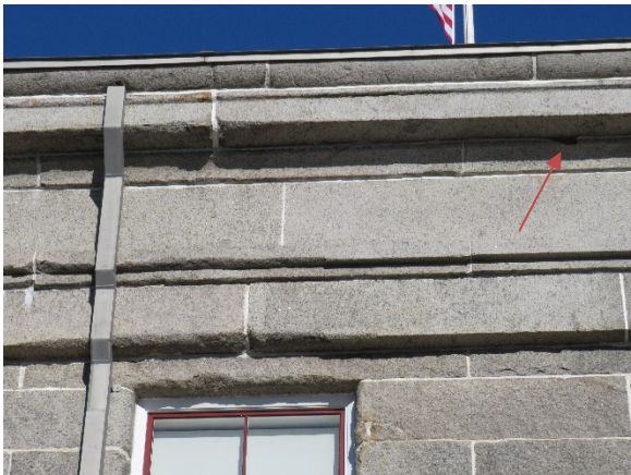
19. East façade, open bed joint above window B2
