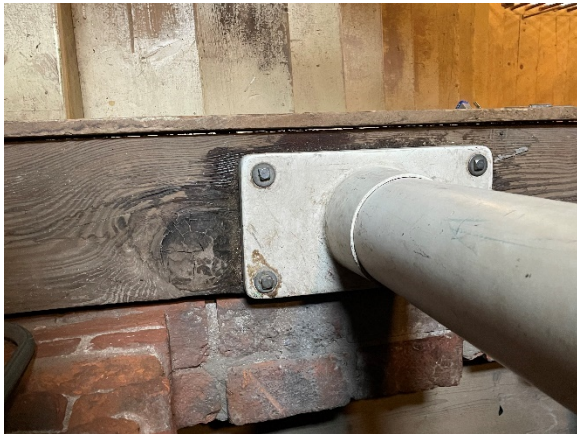
11. Flagpole base with evidence of wetting of the supporting structure. Photo by Joan Whitlow
