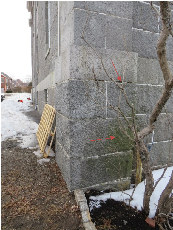
16. Northeast pilaster base – biological growth and mortar loss at ferrous metal setting wedges below watertable
