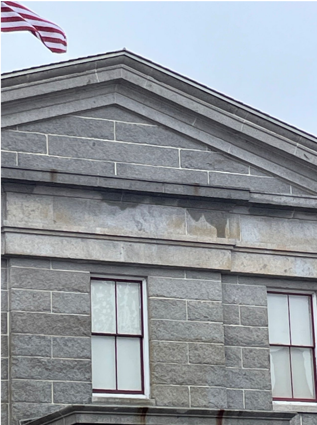
South façade gable bed joint failure 11/16/2022
