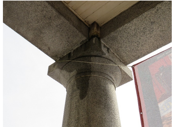
13. Portico southeast column capital with evidence of active water leaking through ceiling
