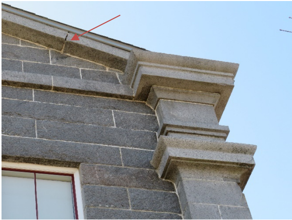
20. North façade, west rake – open mortar joint
