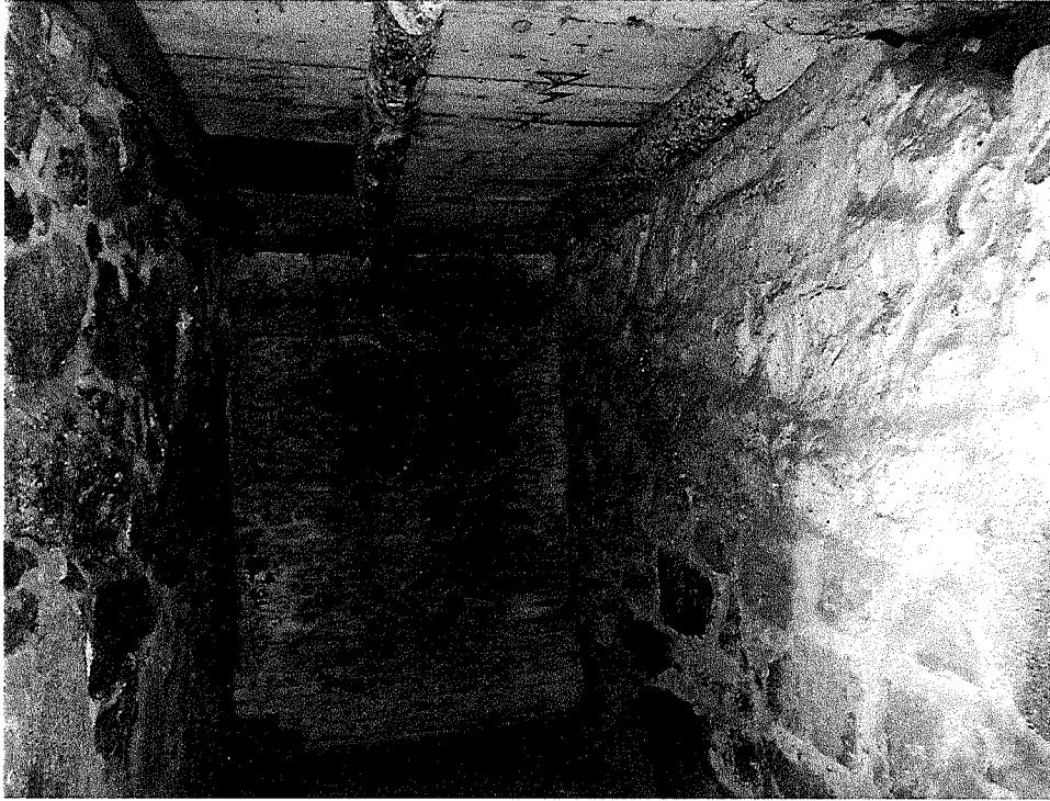
10. Basement condition – June 2015
