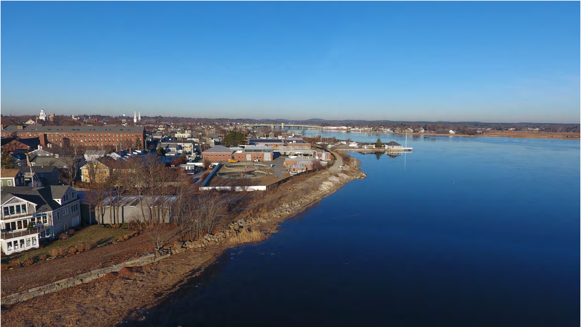
Looking northwest (December 2018) along the Merrimack River shoreline trail corridor towards downtown (note existing granite block seawall transitioning to deteriorated riprap revetment)
