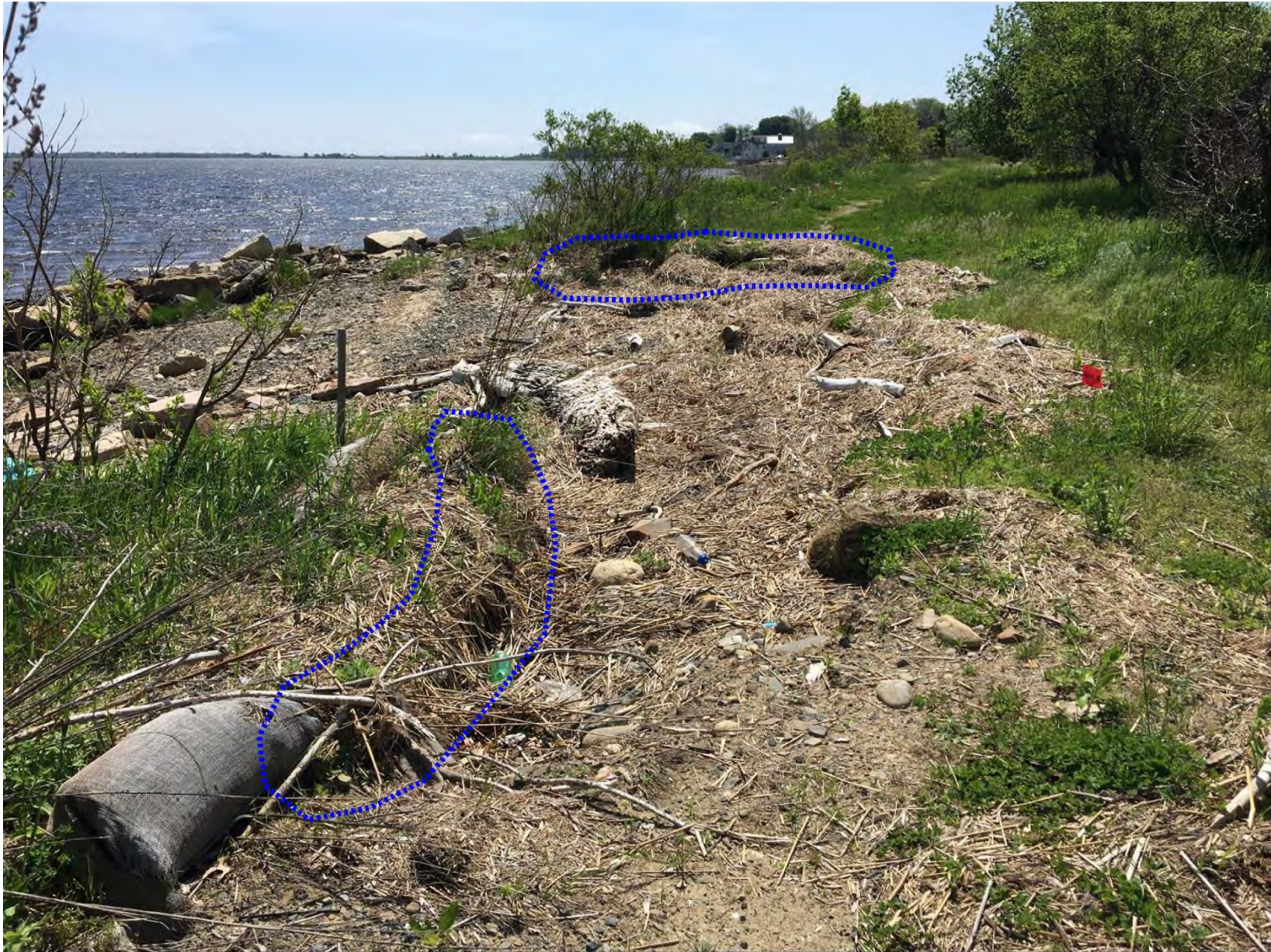
Debris from storm surge across shoreline trail corridor with recently eroded areas circled (May 2018)
