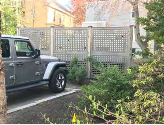
View of generator from the bank parking lot
