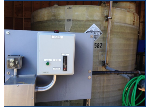
Ferric Chloride Storage Tank
