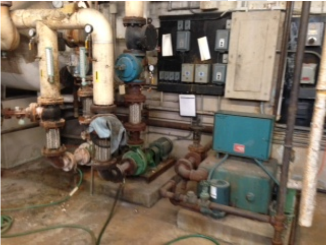
HOT WATER CIRCULATION PUMPS
