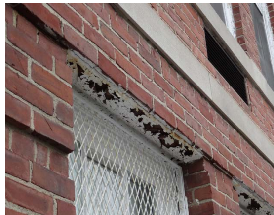
NO CORROSION PROTECTION AT LINTELS
