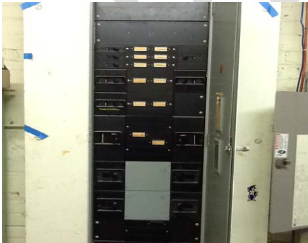
4400 AMP 120/208V-3P MAIN DISTRIBUTION PANEL MAIN SWITCH PUMPS
