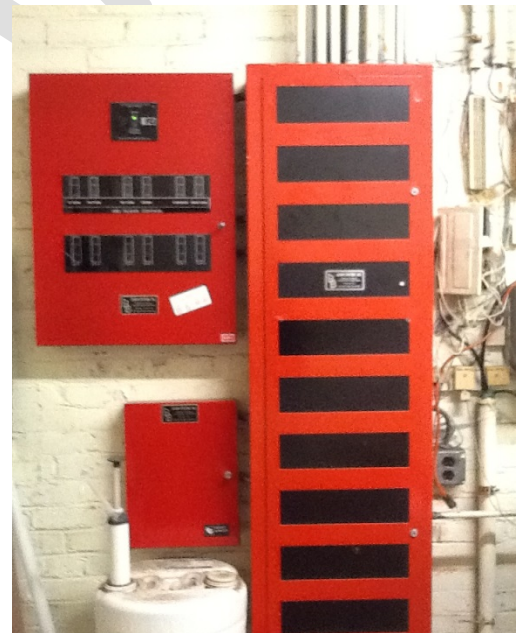
FCI MODEL FC-72 MAIN FIRE ALARM PANEL – LOCATED IN 1ST FL. ELECTRIC ROOM
