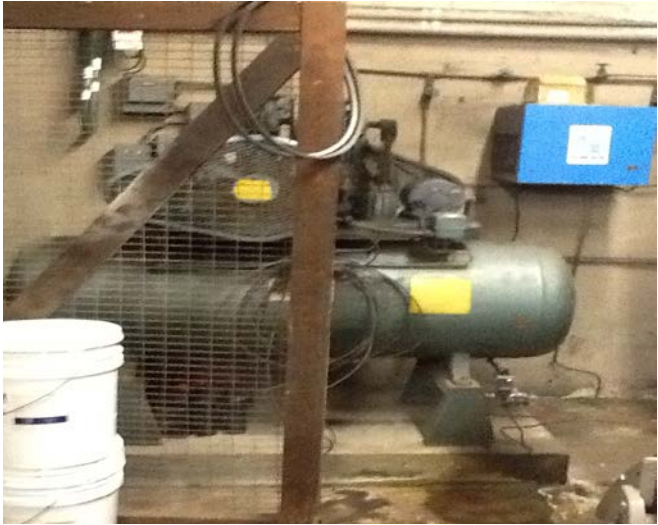
AIR COMPRESSOR FOR PNEUMATIC CONTROLS
