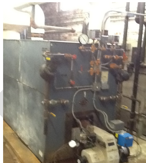
WEIL MCLAIN OIL FIRED BOILER
