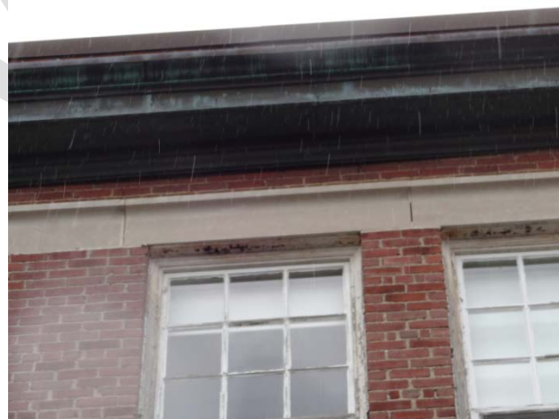
MISSING MORTAR AT HEAD JOINTS
