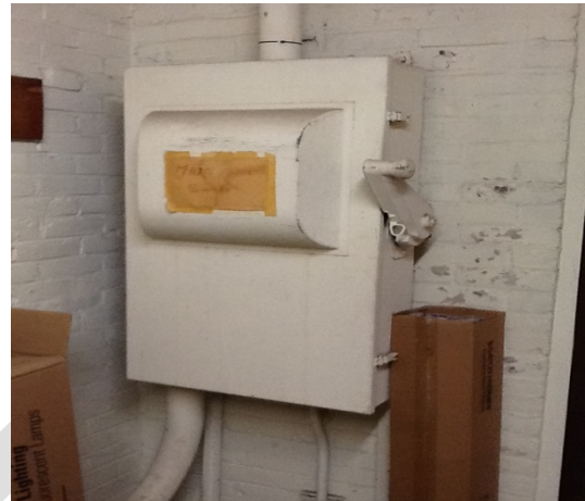
400 AMP 120/208V-3P MAIN SWITCH PUMPS
