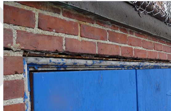
RUSTED JACK LINTELS AT BOILER HEAD HOUSE
