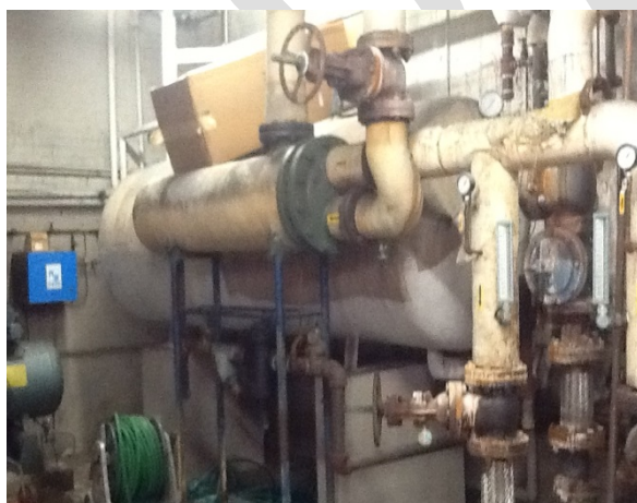
HOT WATER HEAT EXCHANGER
