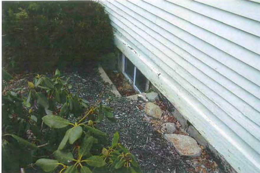
12_View northeast showing principal facade (northwest elevation) - detail of foundation and basement window at north end
