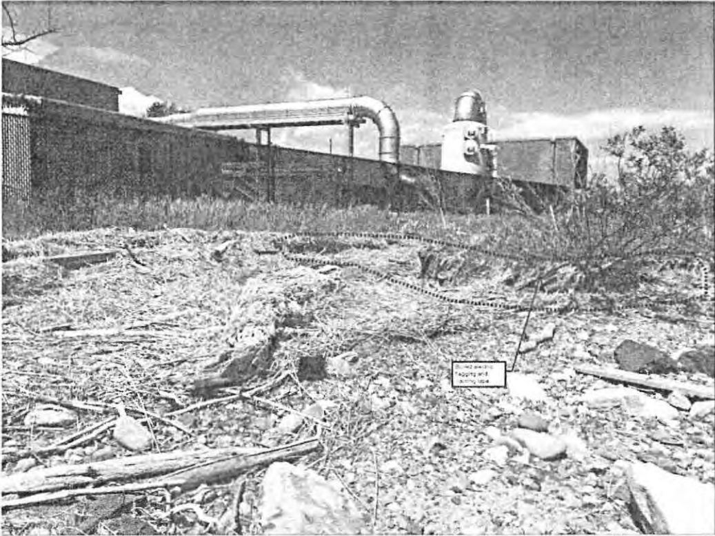
Erosion of shoreline bank (May 2018) – exposed buried electric flagging and warning tape and proximity of underground electric duct bank
