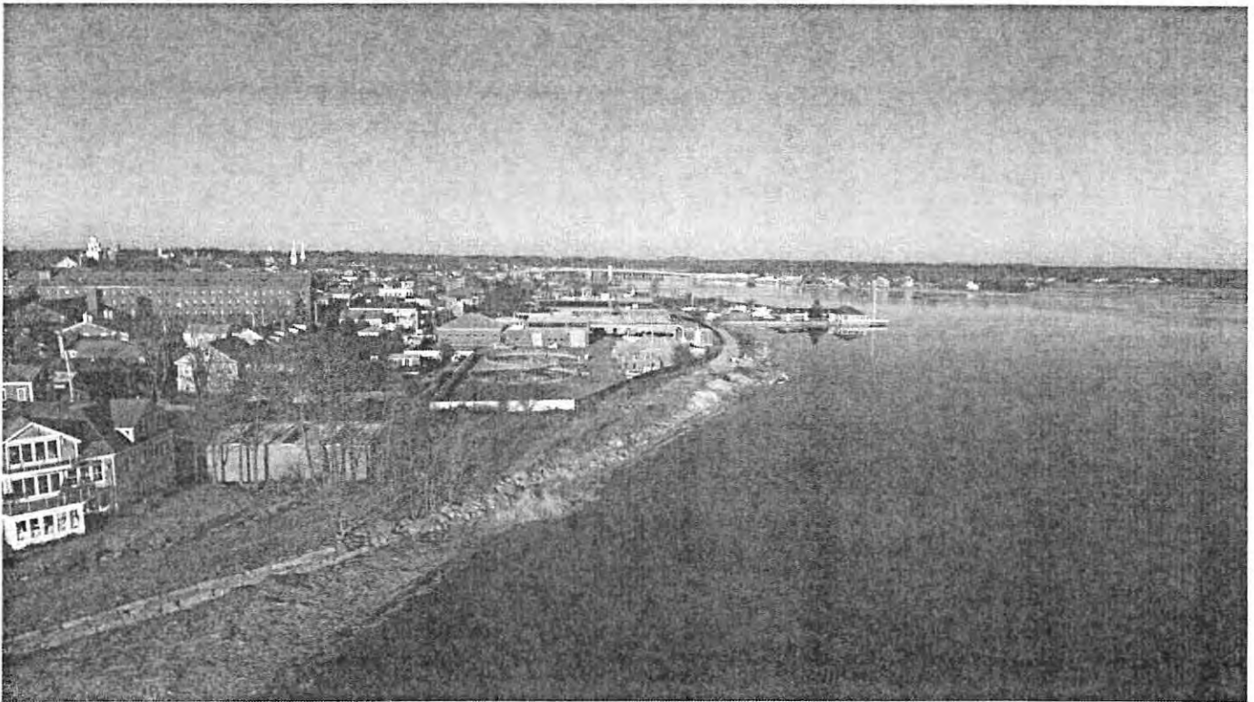
Looking northwest along old rail corridor and WWTF - note deteriorated riprap revetment and temporary shoreline stabilization
