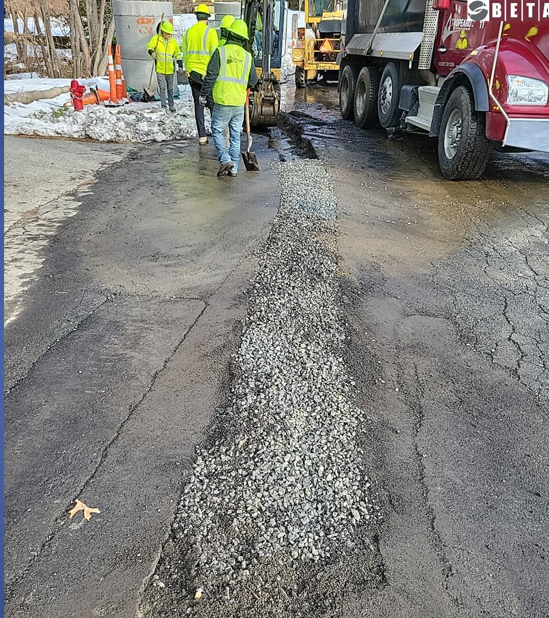
Mar 7, 2023 8:24:31 AM Philips Drive Newburyport, Essex County 01950 Temporary French Drain for Groundwater
