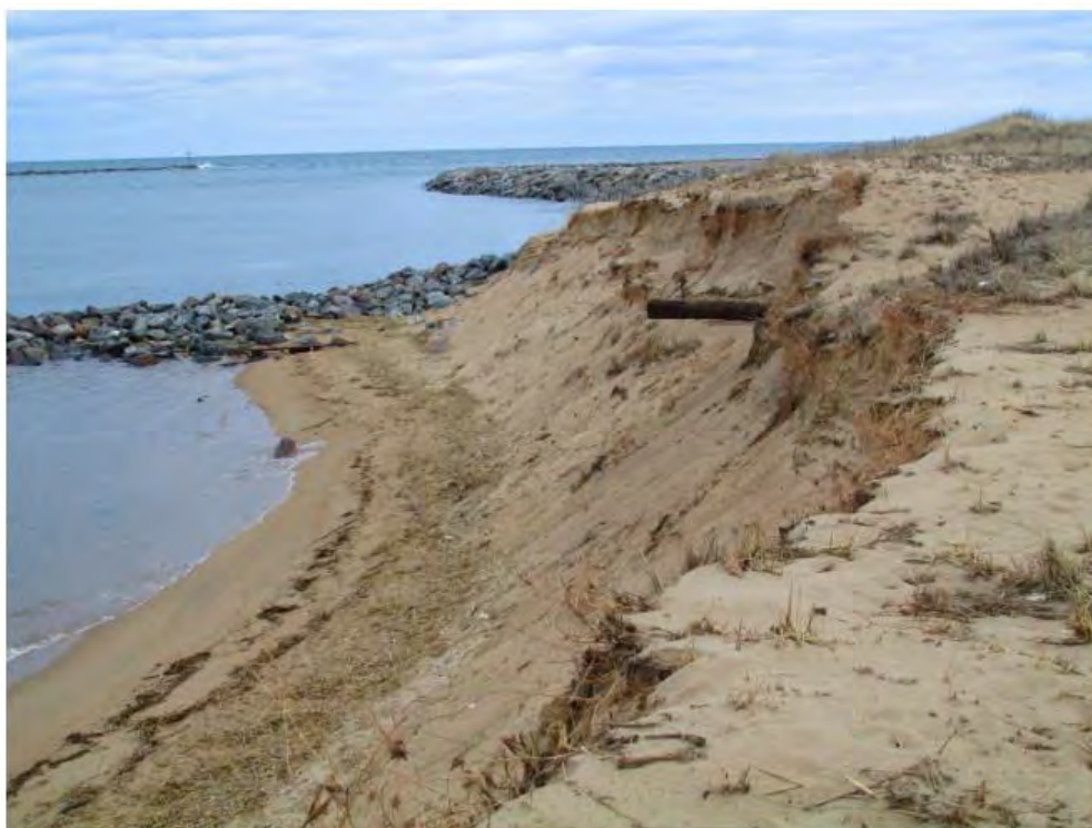
Figure 4.1.2 Coastal Erosion in Newburyport. Photo credit: Sandy Tilton, Great Marsh Coastal Adaptation Plan (2017).
