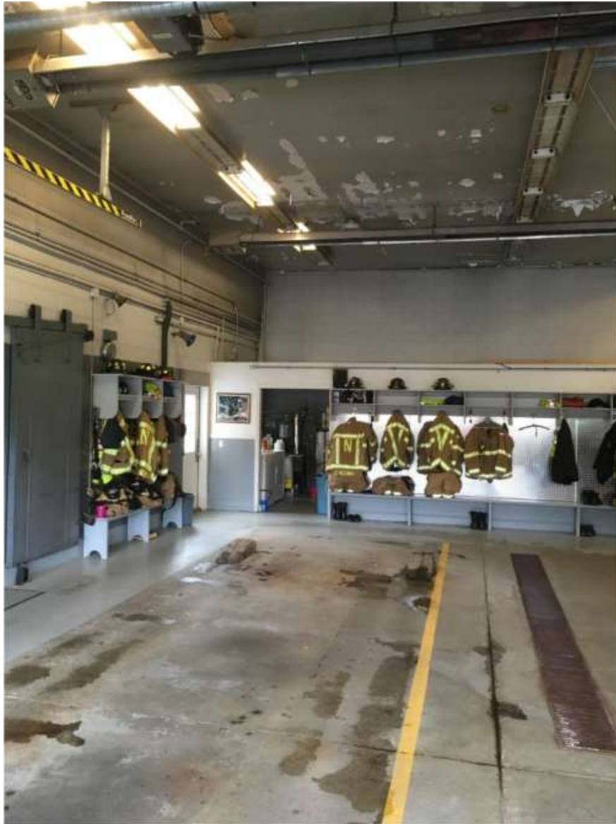
• Energy inefficient lighting
