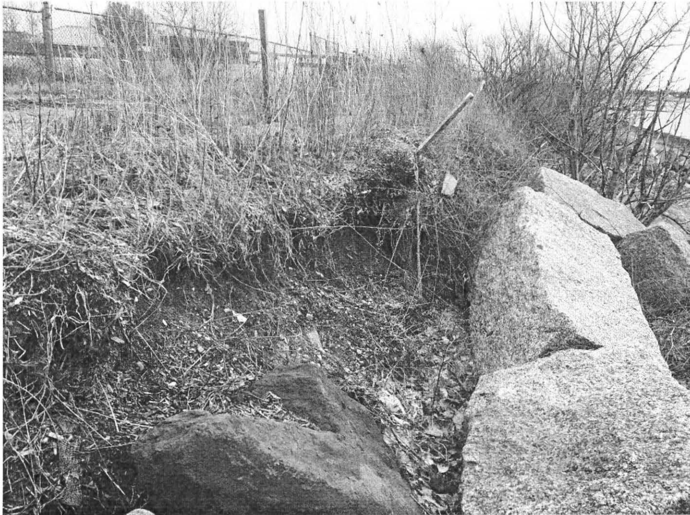
New erosion above old stabilization rip rap (April 2020)
