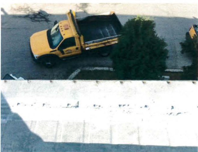
Rusted fasteners at rake trim - should be stainless steel fasteners.
