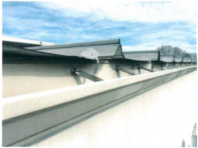
Standard K-style aluminum gutters and hangers - original metal gutter system must have been replaced
