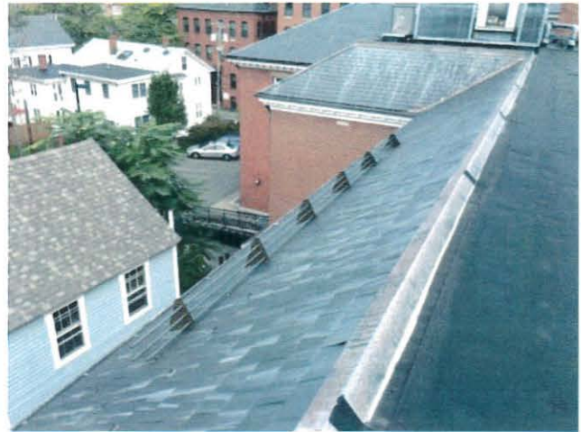
Damaged snow fence at the northwest side
