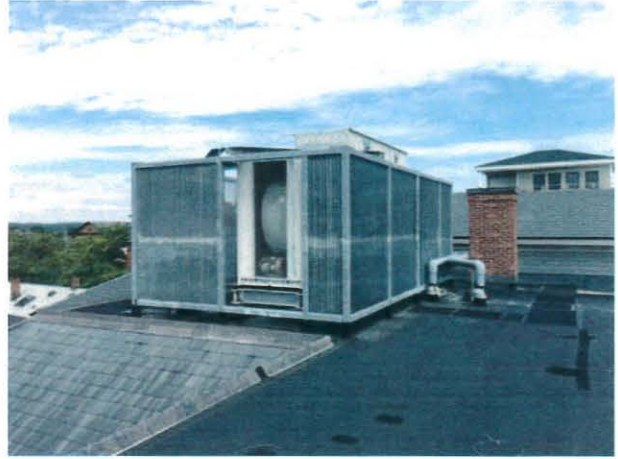
Equipment Screen at Mechanical Unit
