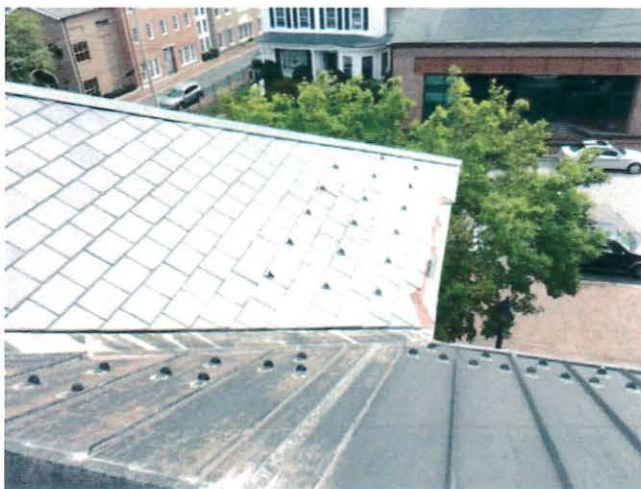
Damaged and missing slate shingles at original building roof
