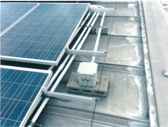
Concrete blocks used as rooftop supports at equipment directly on metal roof
