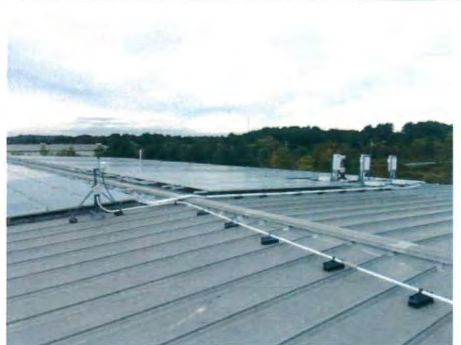
Solar photovoltaic system equipment & cabling - cabling should be secured to roof panels
