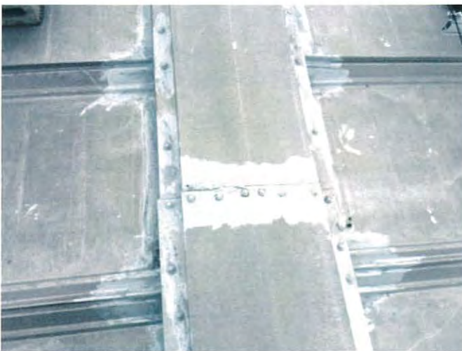
Seam repairs at ridge caps - fasteners are backing out and many do not have EPDM washers
