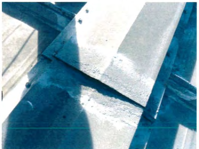
Open seams at ridge cap - no fasteners
