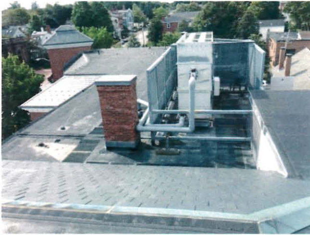
Looking southwest at Mechanical Unit
