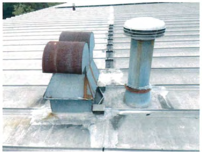
Flashing repairs at various roof penetrations - curbs appear to have been installed after the roof was completed
