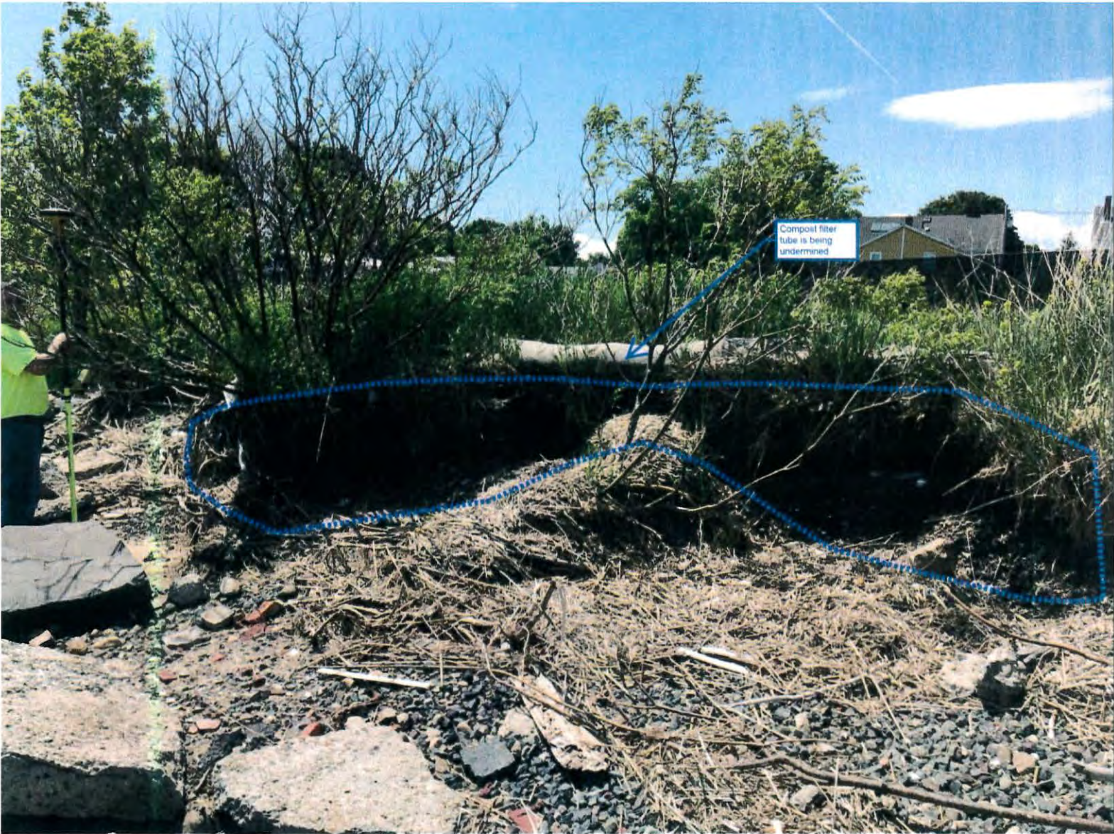
Scoured river bank of shoreline trail corridor in May 2018 (recently eroded area circled)
