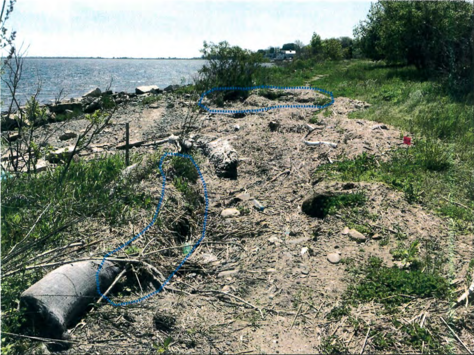
Debris from storm surge across shoreline trail corridor with recently eroded areas circled (May 2018)
