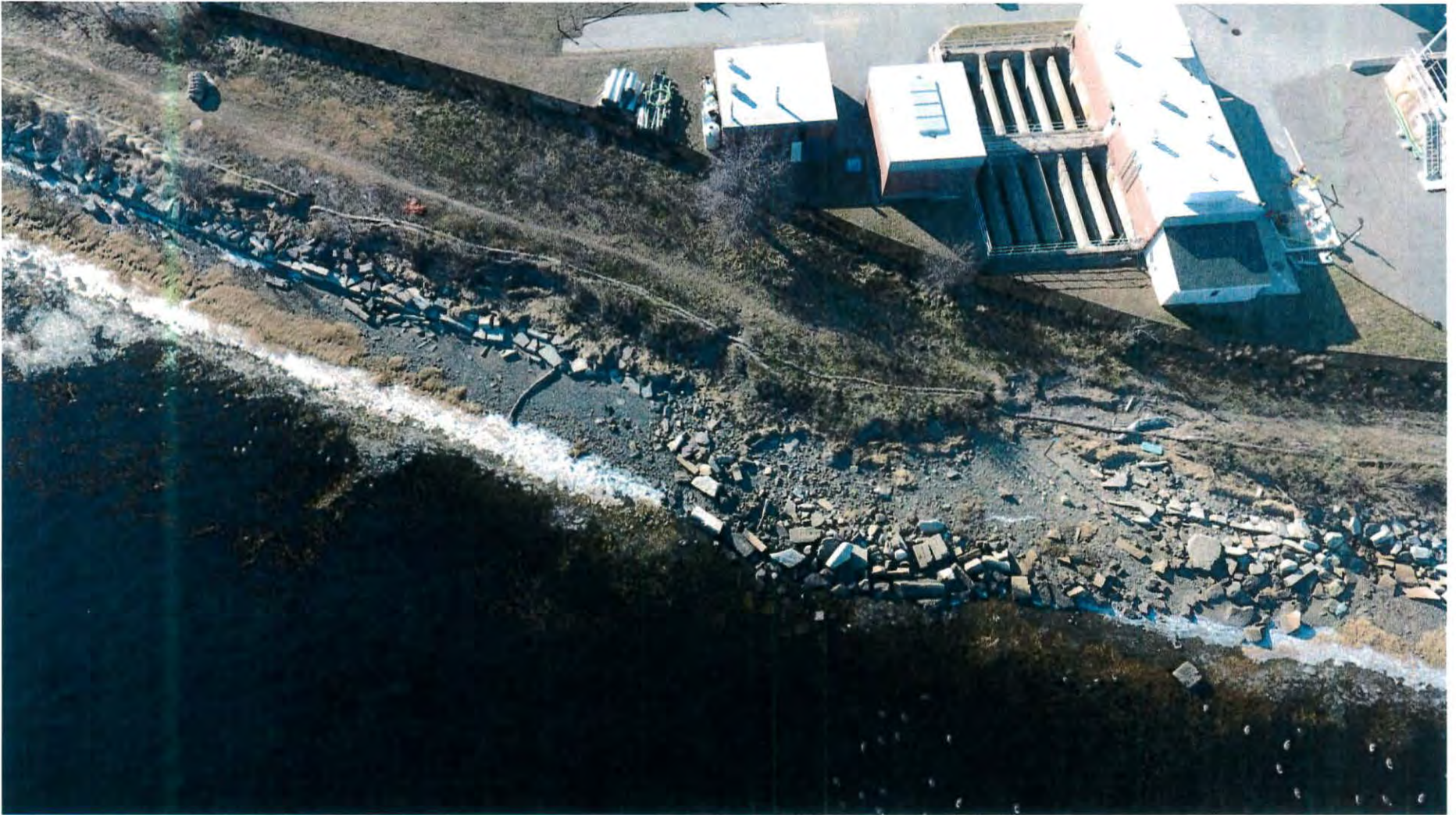
Aerial photo (December 2018) of portion of scoured shoreline along riverfront trail corridor
