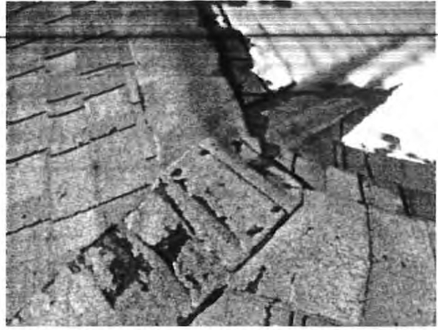
Deteriorated shingles at intersection of hip, valley & ridge
