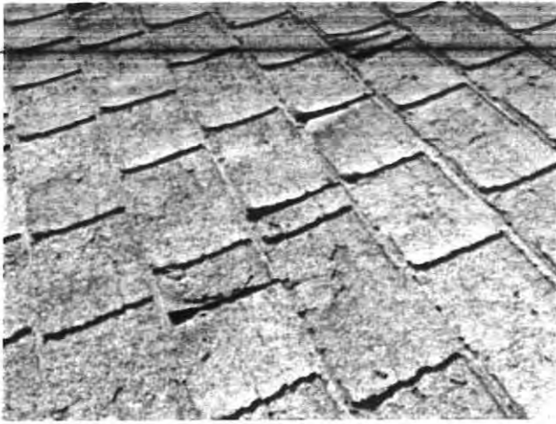
Deteriorated shingles - granule loss & curling
