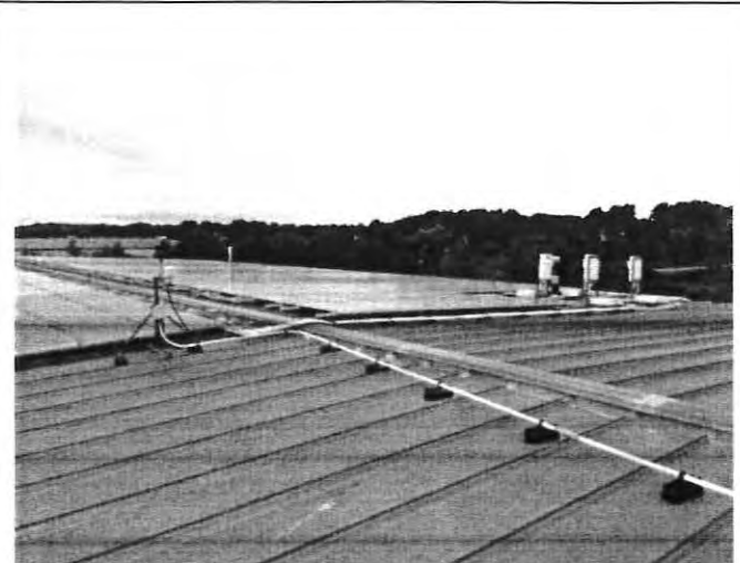
Solar photovoltaic system equipment & cabling - cabling should be secured to roof panels
