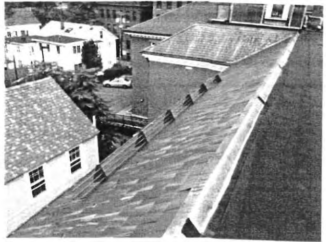
Damaged snow fence at the northwest side
