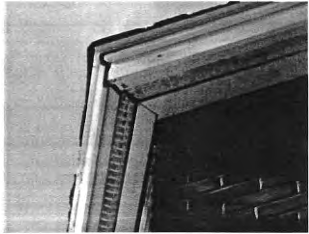
Deteriorated fascia boards and soffits
